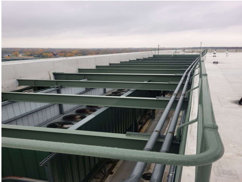
Photo A.4a — Roof looking north along the chiller pit opening. Structural steel bays span the top of the pit at roof level. The open bay with condenser fans visible below is the proposed location for the new Phase 2 chiller. Structural steel is existing and pre-installed in Lambeau Green paint to match.
