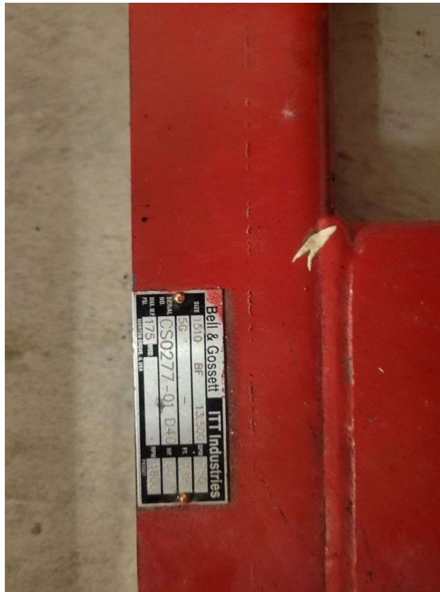
Photo A.3a — Bell & Gossett ITT Industries pump. Size 1510, BF 13,500 GPM, Serial CS0277-01 D40, 175 PSI max WP. Original vintage pump — no VFD.
