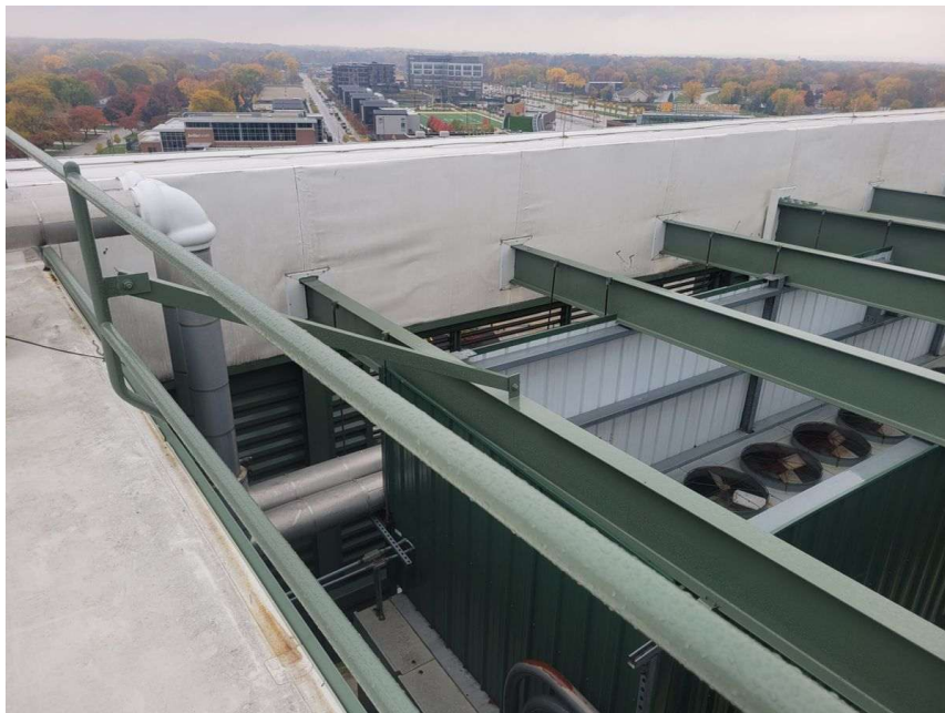
Photo A.4c — Roof level view showing open structural bay and existing piping headers below in the pit corridor. This bay view illustrates the available space for new chiller placement during Phase 2 and demonstrates the direct crane access from above.
