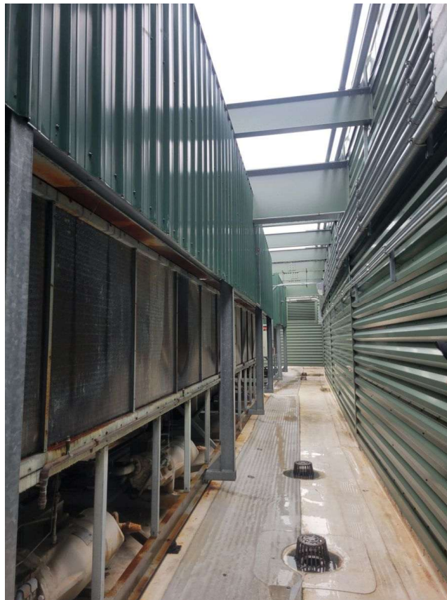
Photo A.1a — Pit corridor looking north. Chiller condenser frames (left) show structural rust on base rails and fin deterioration. The narrow width of the pit relative to chiller height restricts discharge air clearance, driving recirculation.
