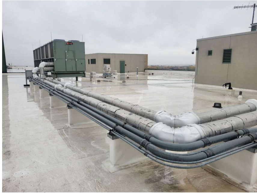
Photo A.4d — Existing Chiller 3 (Trane Series R) installed at roof level, viewed from the main roof deck. Insulated chilled water supply and return piping runs from the unit across the roof on pipe supports. This installation validates the roof chiller concept — Phase 1 will replace this unit in-kind with a new 500-ton Trane chiller.
