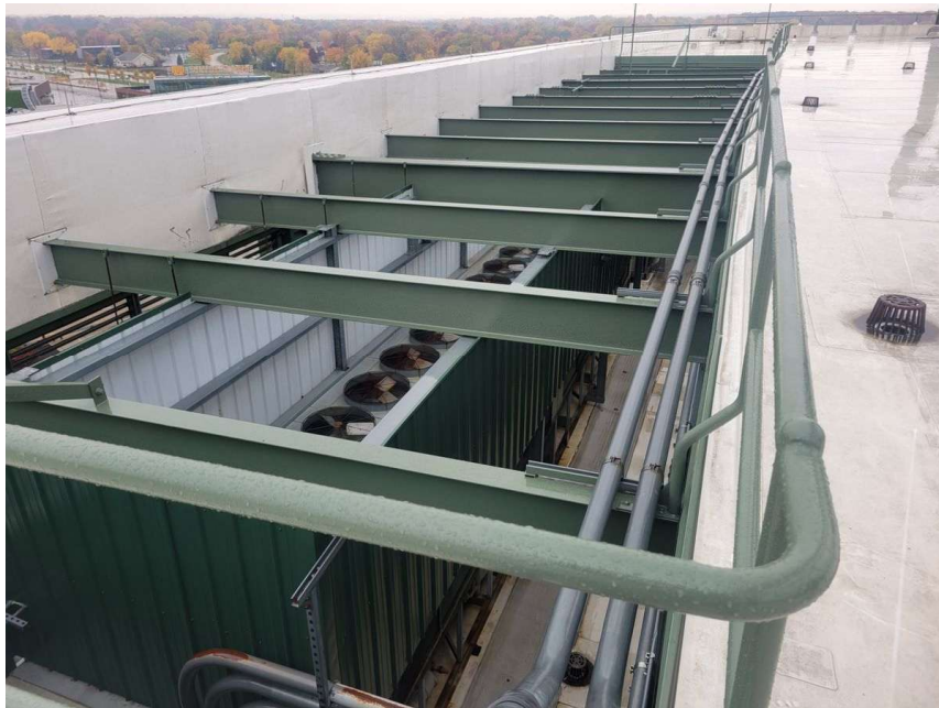
Photo A.4b — Roof view showing multiple structural bays above the pit. Condenser fan arrays of the existing chillers visible below in each bay. The open sky above each bay confirms unrestricted discharge air clearance — no recirculation when equipment is repositioned at this elevation.
