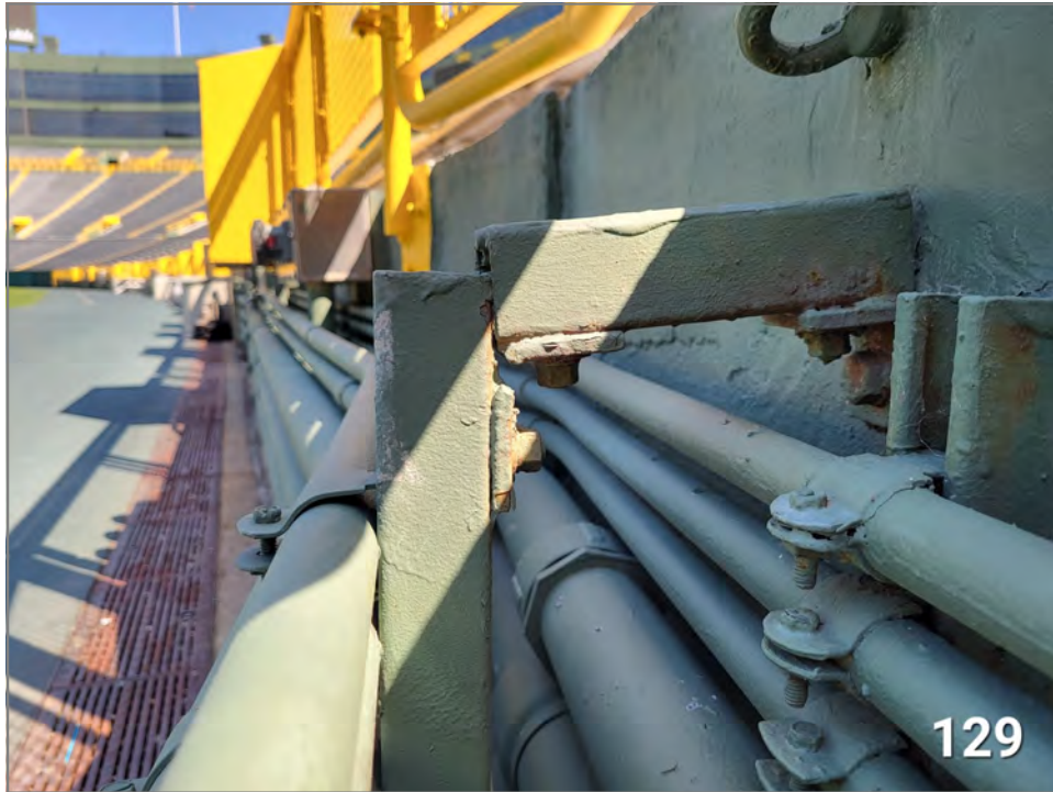
Bowl and Seating: Photo 1-1-5 Sealant failing
