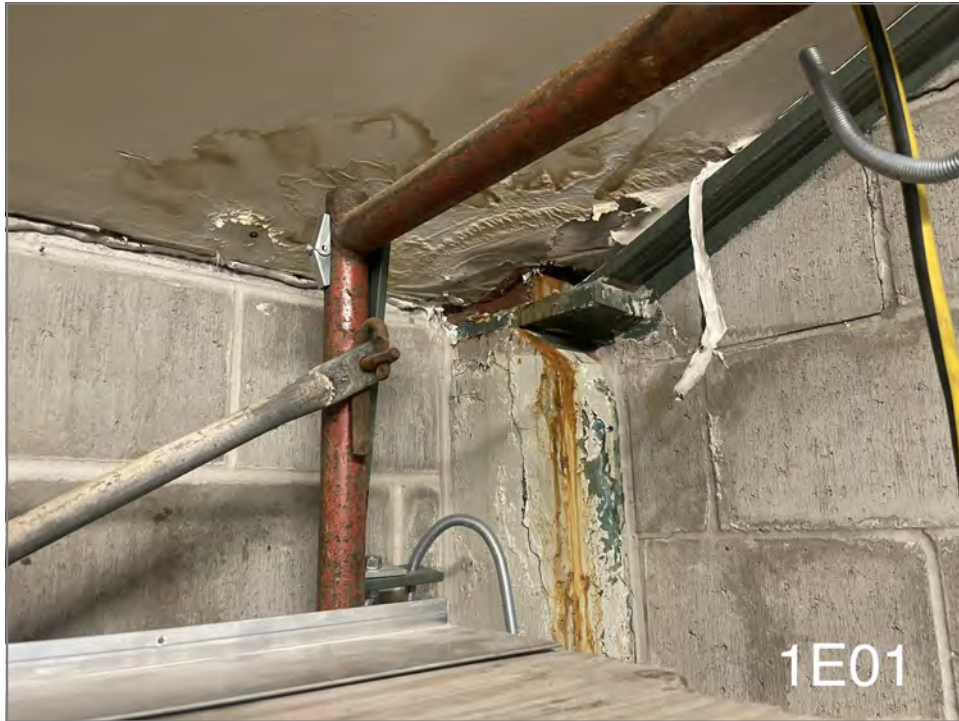
Interior and Finishes: Photo 4- -3 Water damage
