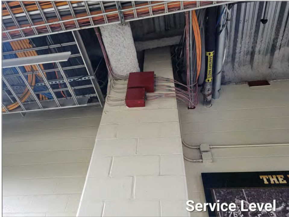
Concourses: Photo 2-0-3 Paint peeling
