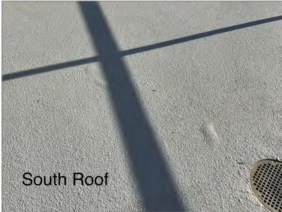
Roof: Photo 6- -37 Traffic membrane lifting
