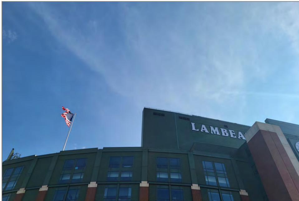
Exterior Walls: Photo 5- -9 Window seal broken
