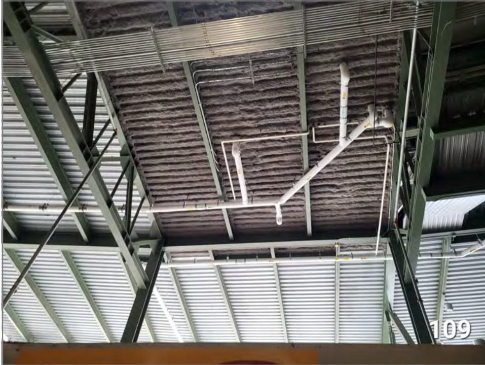
Concourses: Photo 2-100-8 Missing saddle plates
