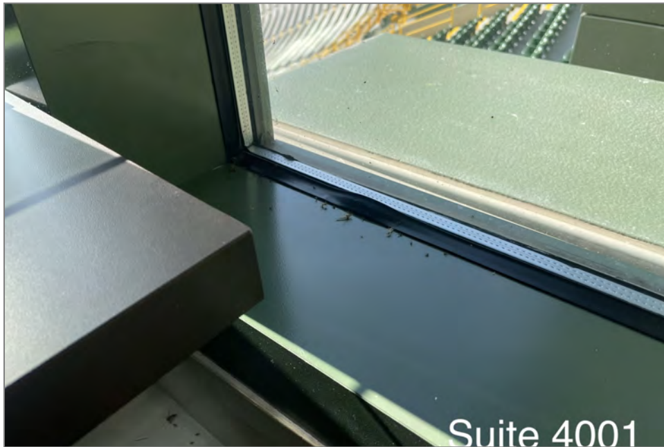
Interior and Finishes: Photo 4-4-26 Window frame seal failing
