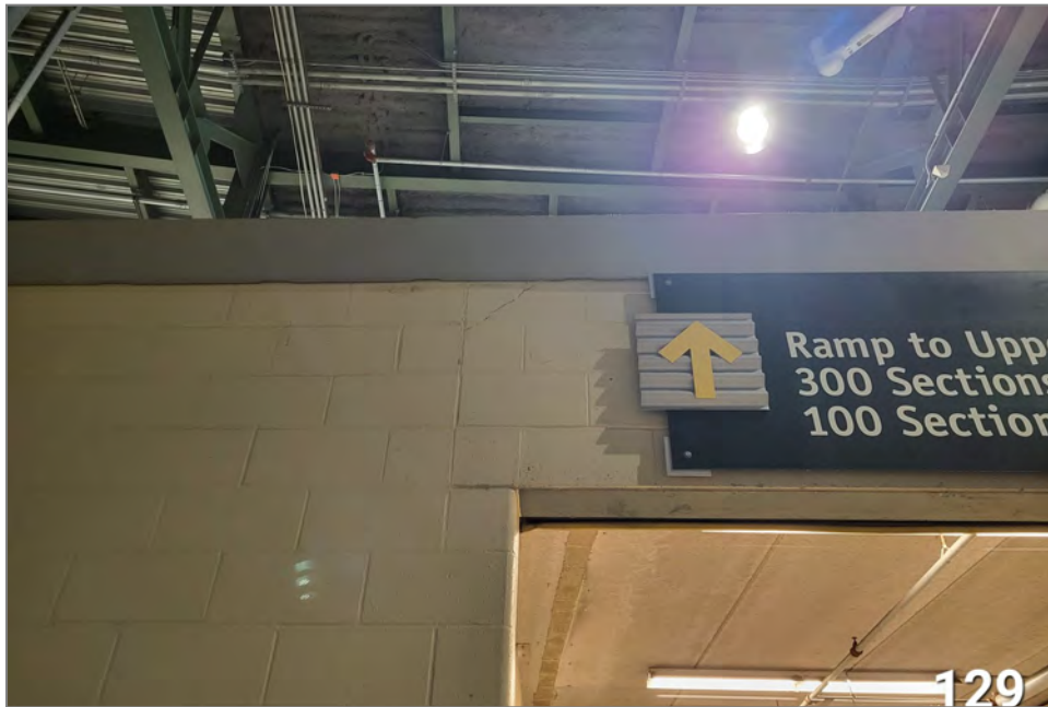
Concourses: Photo 2-100-1 Block cracking
