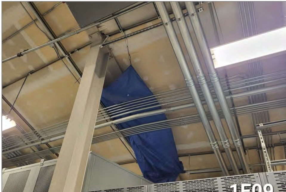
Interior and Finishes: Photo 4- - 13 Water damage
