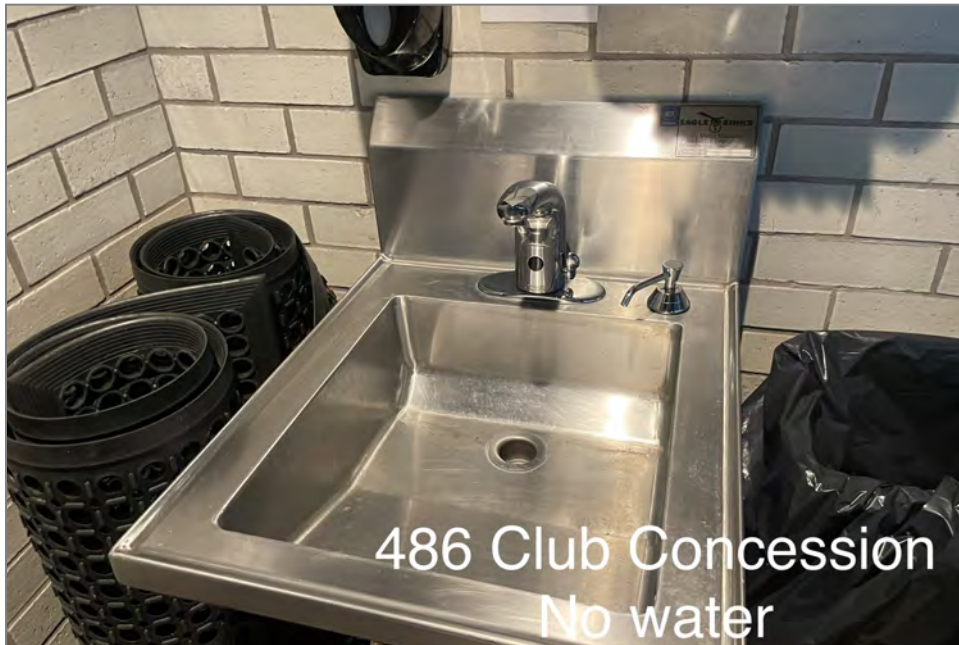
Concessions: Photo 3- - 23 No water from sink
