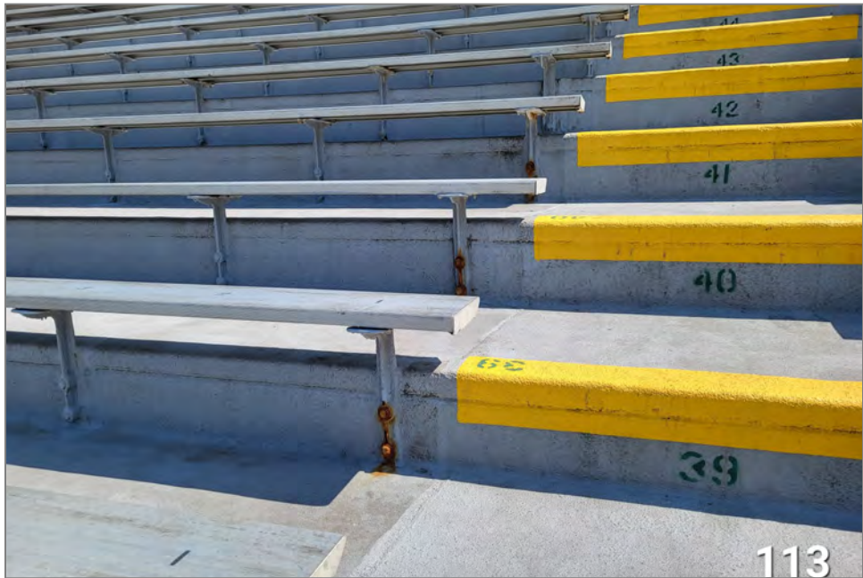
Bowl and Seating: Photo 1-2-1 Bleacher support corroding
