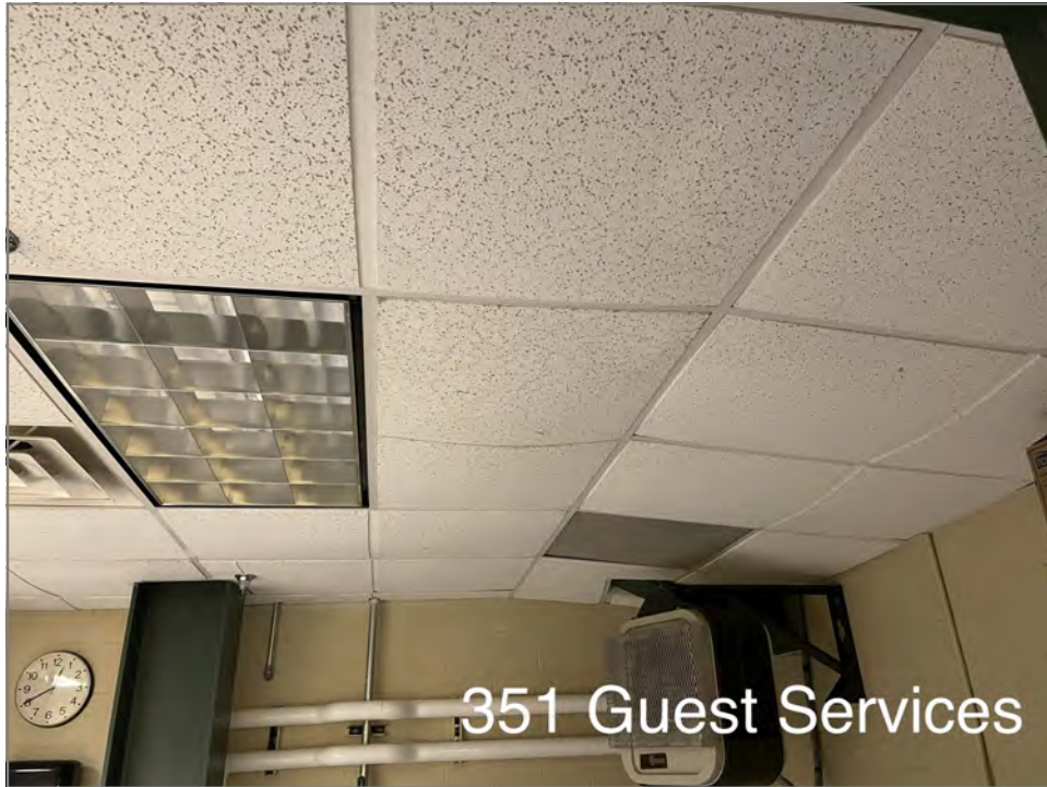
Interior and Finishes: Photo 4- -8 Sagging drop ceiling grid
