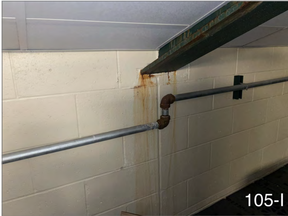
Concessions: Photo 3- -10 Structural steel corrosion
