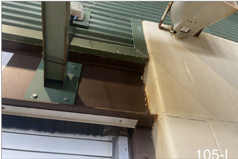
Concessions: Photo 3- -11 Structural steel corrosion
