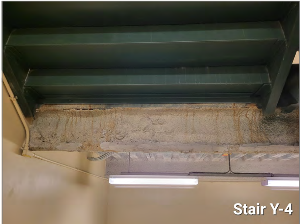
Interior and Finishes: Photo 4-3-4 Floor pan corrosion
