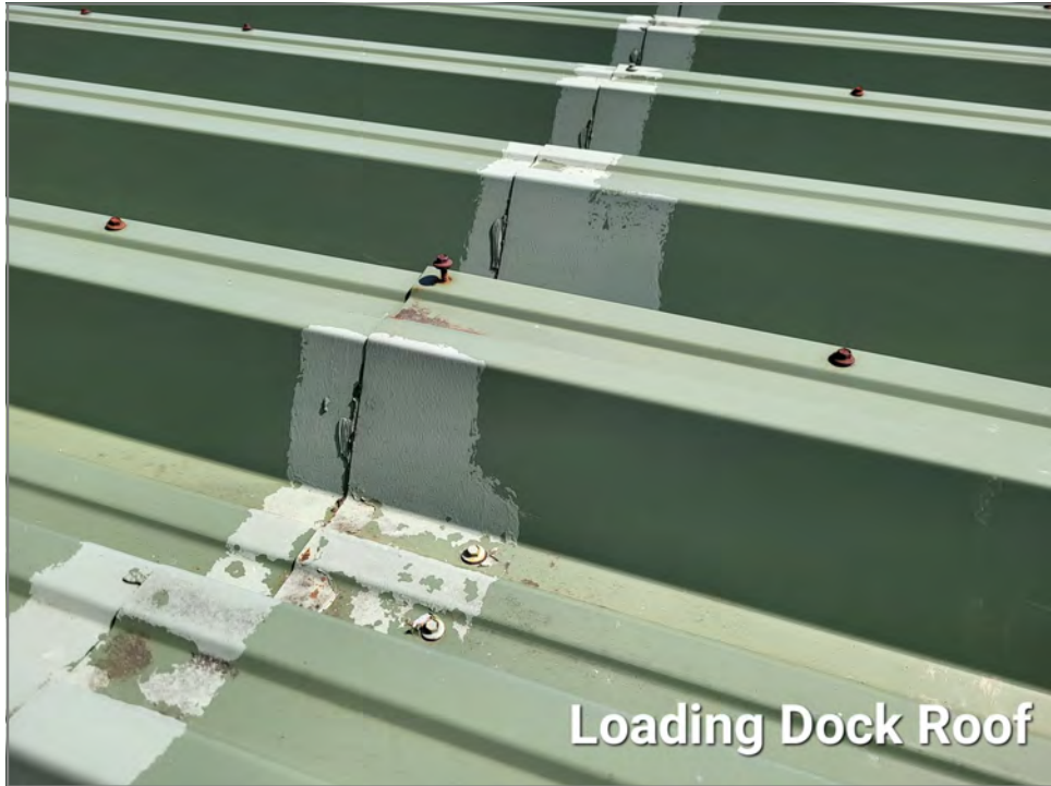
Roof: Photo 6- -3 Loose/backing out fastener
