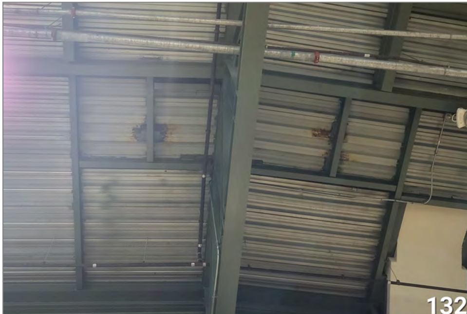
Concourses: Photo 2-100-21 Floor pan corroding
