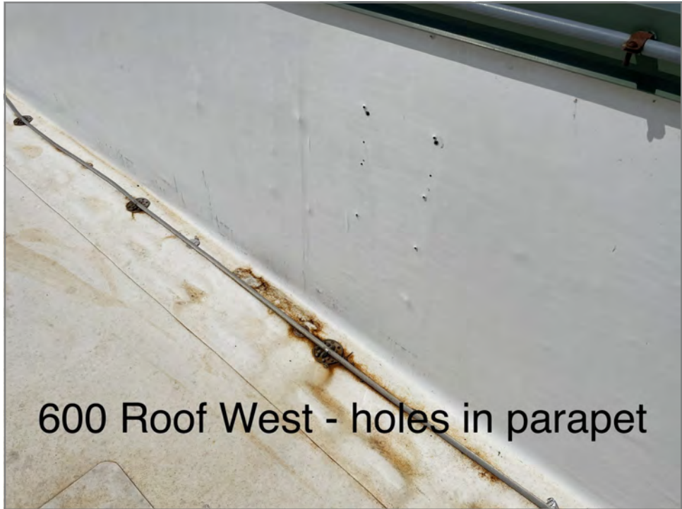
Roof: Photo 6- -35 Membrane cut/open
