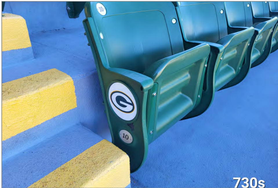
Bowl and Seating: Photo 1-2-32 Paint peeling/cracking or bubbling
