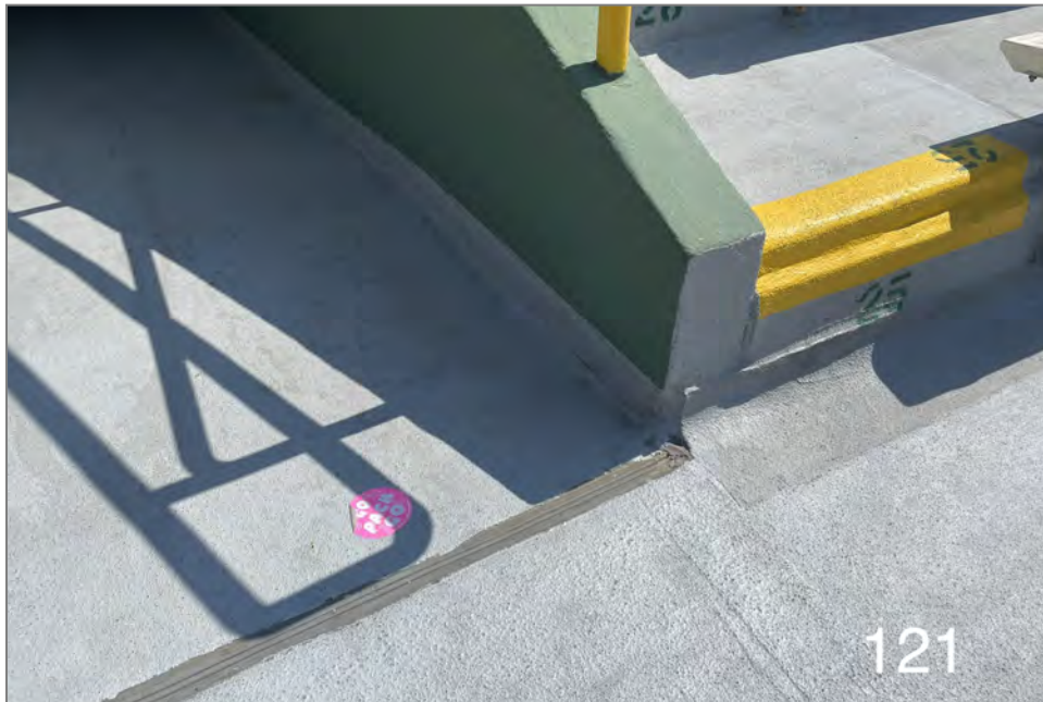
Bowl and Seating: Photo 1-2-73 Exposed expansion joint
