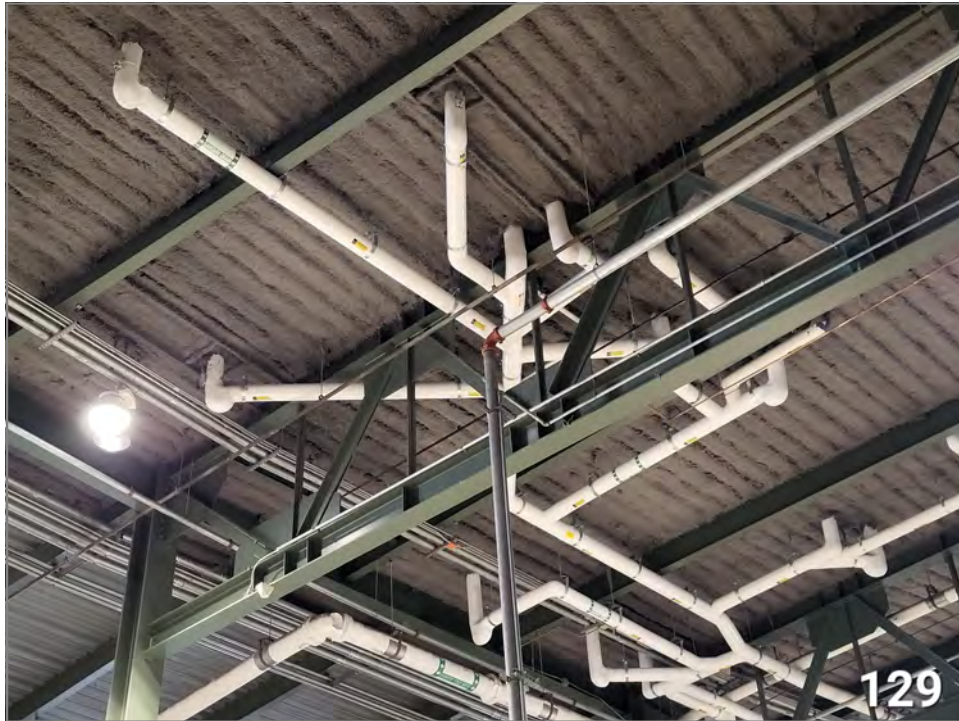
Concourses: Photo 2-100-3 Missing saddle plates
