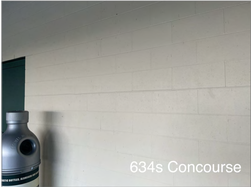
Concourses: Photo 2-600-6 Block cracking
