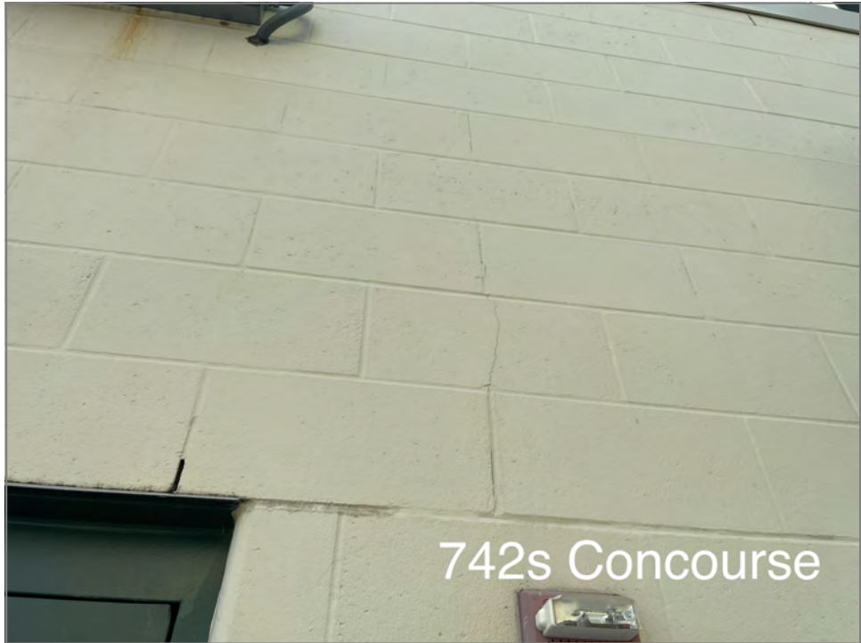
Concourses: Photo 2-700-7 Block cracking
