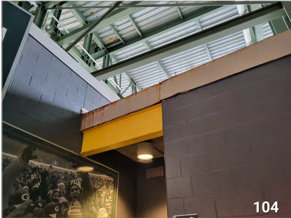
Concourses: Photo 2-100-12 Flashing corroding
