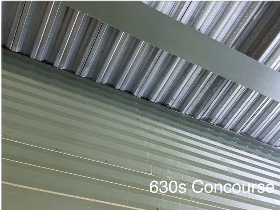
Concourses: Photo 2-600-4 Corroding floor pan
