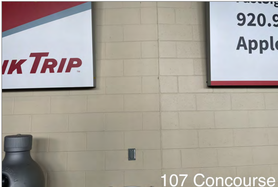
Concourses: Photo 2-100-31 Sealant failing
