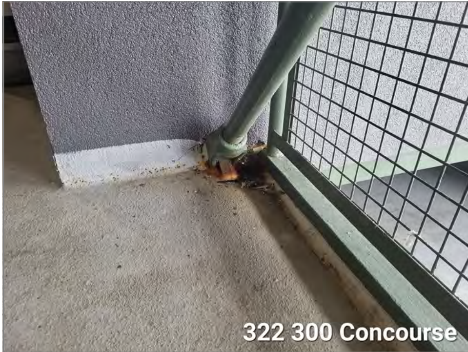
Concourses: Photo 2-300-7 Structural steel corrosion
