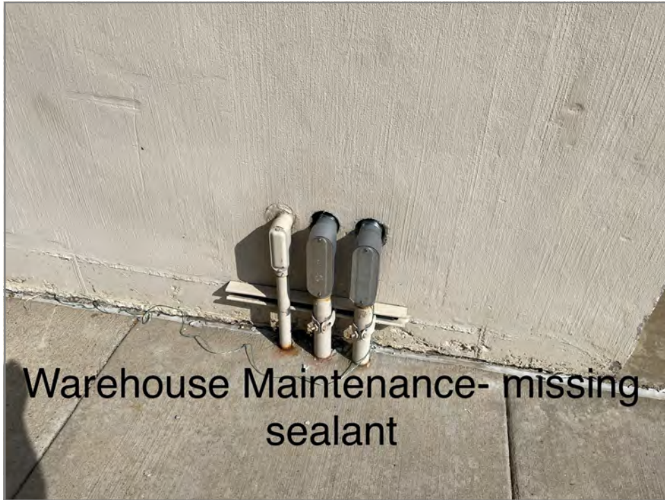
Exterior Walls: Photo 5- -11 Missing/failing sealant
