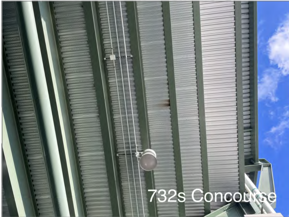
Concourses: Photo 2-700-2 Corroding floor pan
