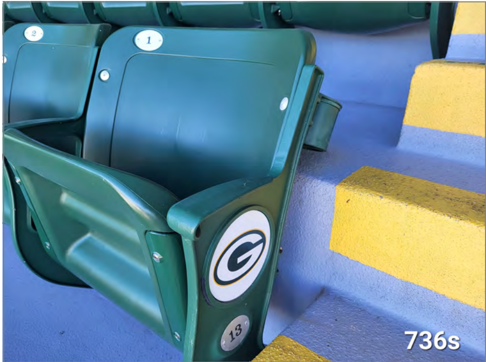
Bowl and Seating: Photo 1-2-33 Paint peeling/cracking or bubbling
