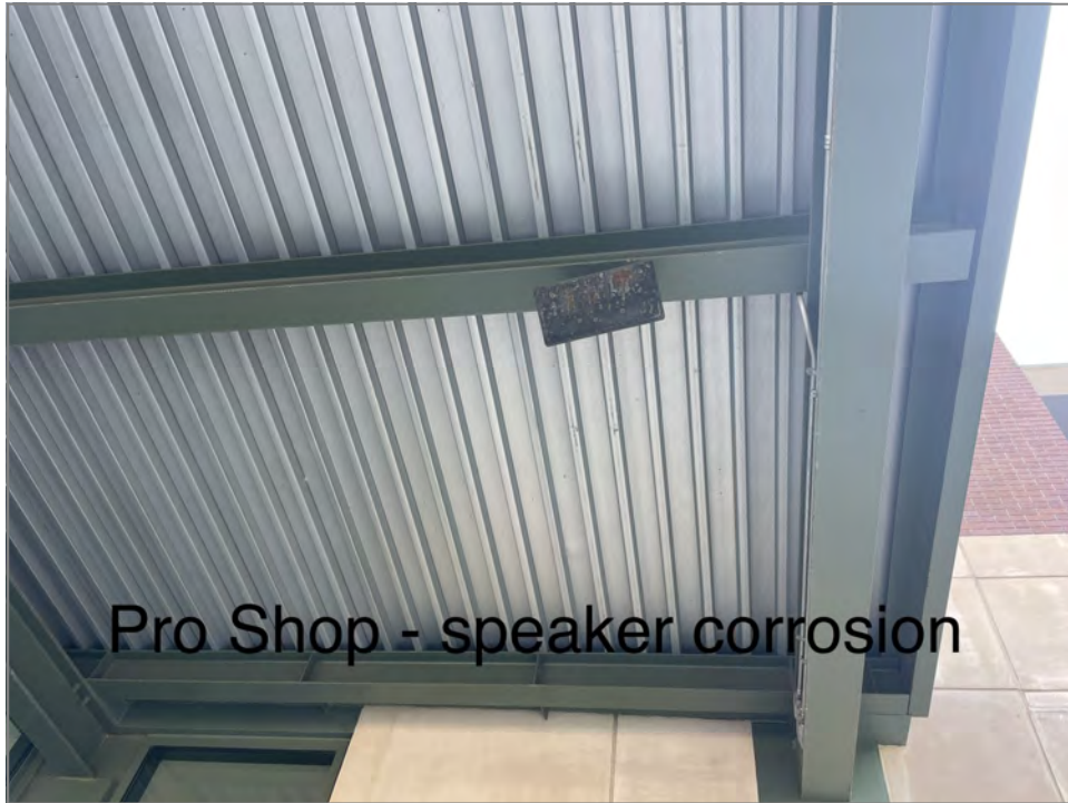
Exterior Walls: Photo 5- -27 Exterior speaker corrosion
