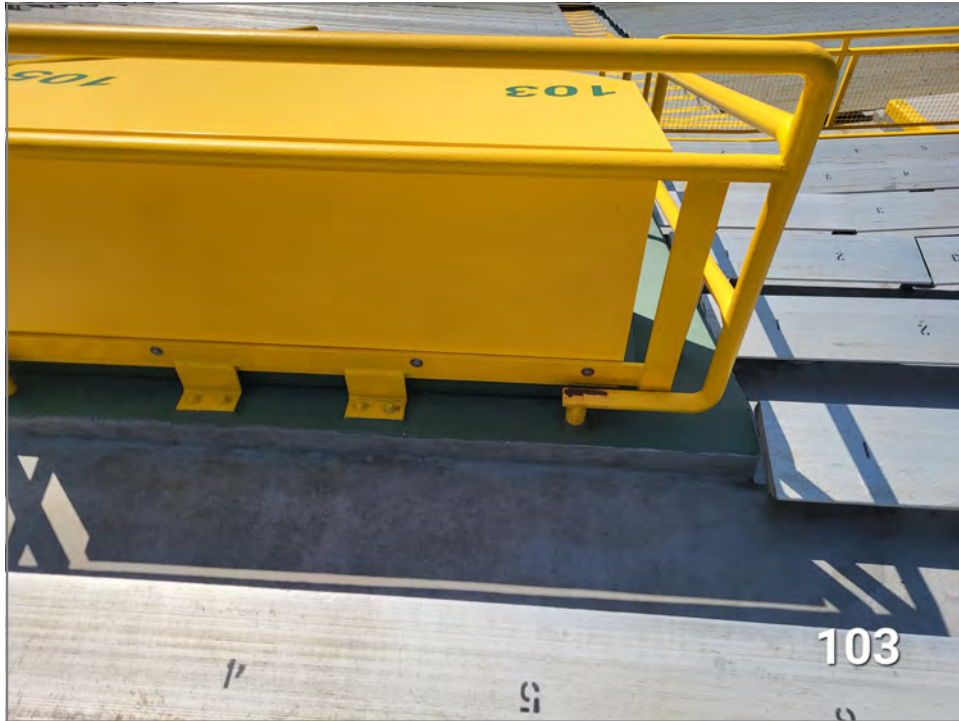
Bowl and Seating: Photo 1-2-4 Handrail and base corrosion
