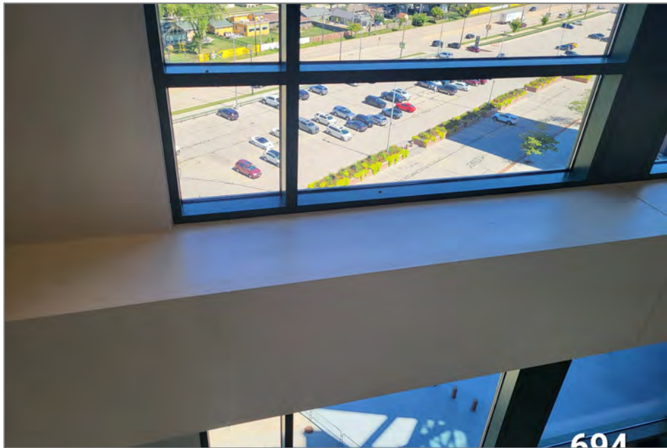
Concourses: Photo 2-600-2 Water damage on interior window sill
