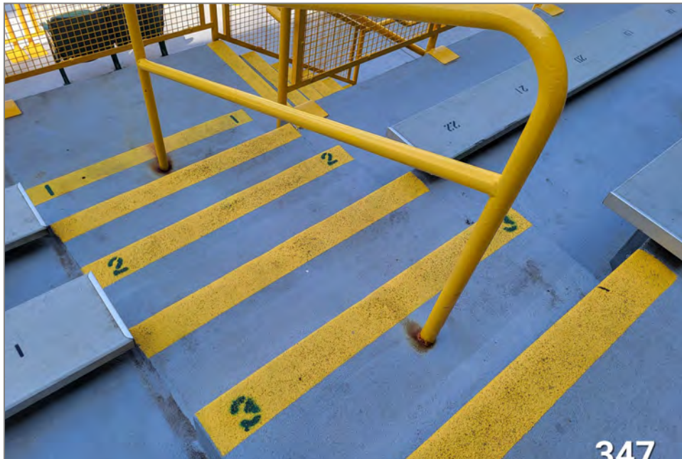
Bowl and Seating: Photo 1-2-15 Handrail and base corrosion
