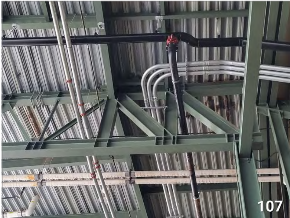
Concourses: Photo 2-100-10 Floor pan corroding
