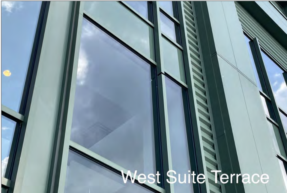
Exterior Walls: Photo 5- -35 Mullions shifting/misaligned
