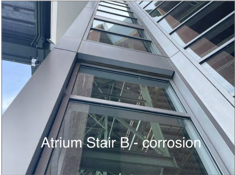
Exterior Walls: Photo 5- -25 Corrosion
