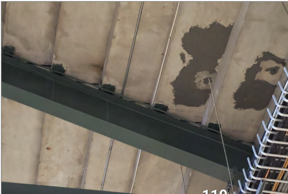
Concourses: Photo 2-100-27 Precast concrete spalling
