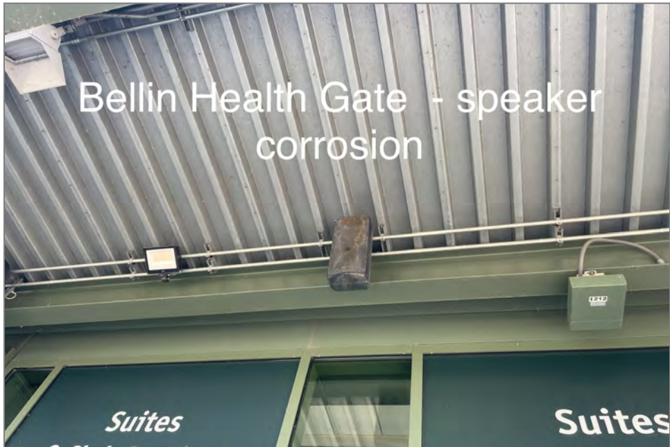
Exterior Walls: Photo 5- -21 Exterior speaker corrosion
