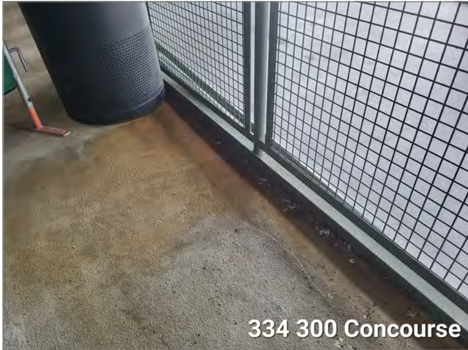
Concourses: Photo 2-300-5 Handrail and base corrosion
