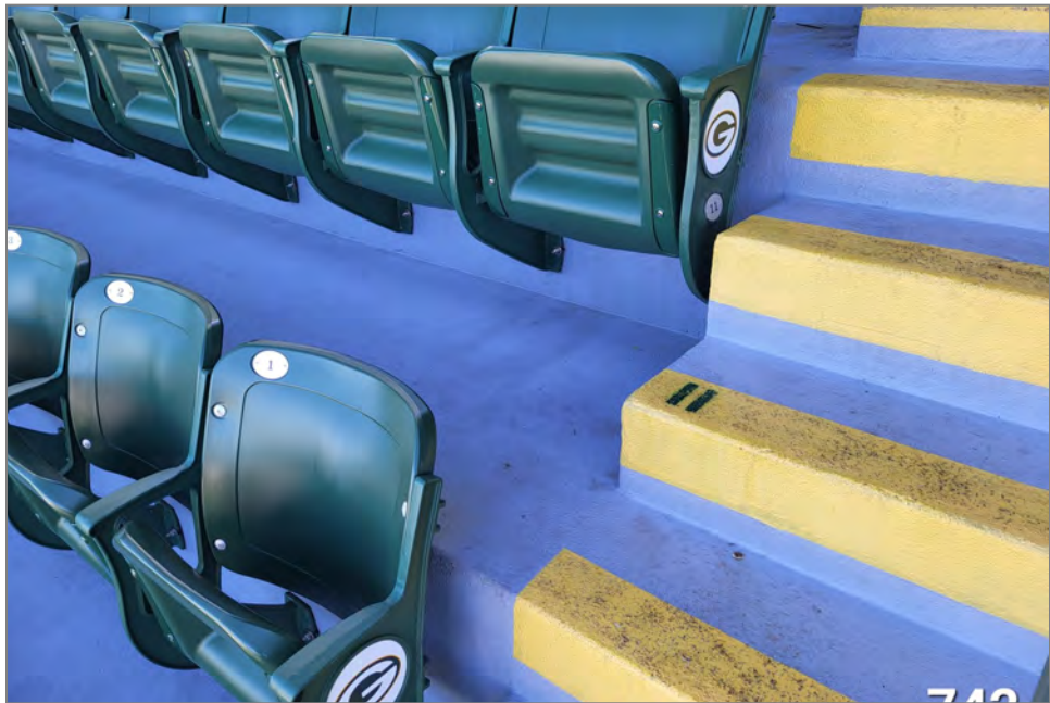
Bowl and Seating: Photo 1-2-34 Paint peeling/cracking or bubbling
