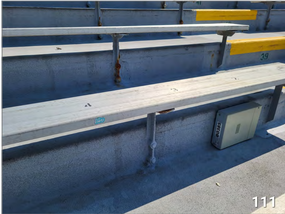
Bowl and Seating: Photo 1-2-2 Bleacher support corroding
