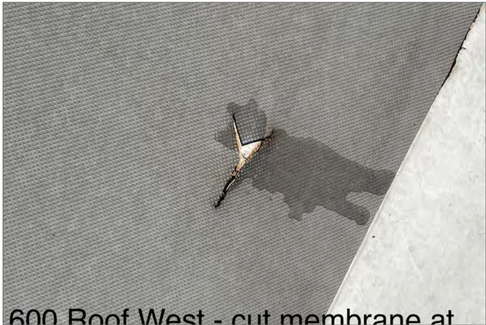
Roof: Photo 6- -34 Membrane cut/open
