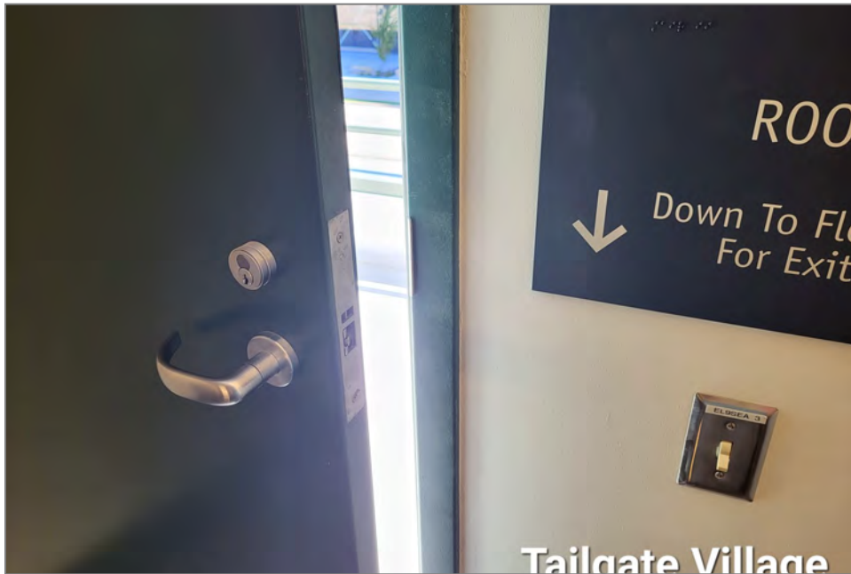
Site: Photo 10-1-3 Door won't close automatically
