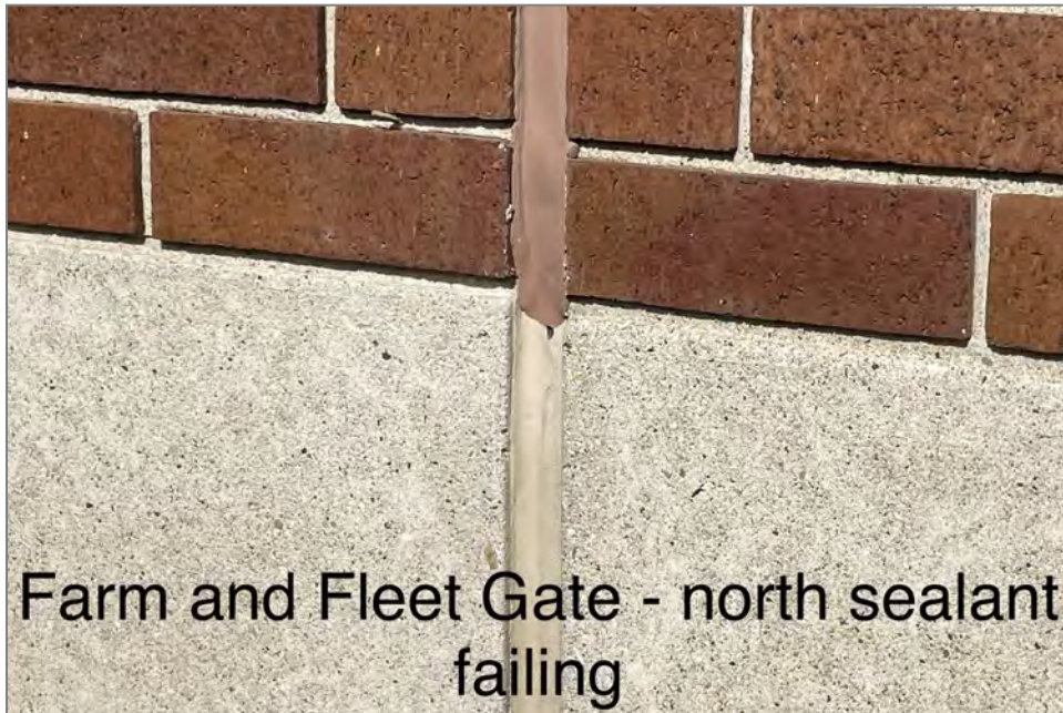
Exterior Walls: Photo 5- -15 Missing/failing sealant
