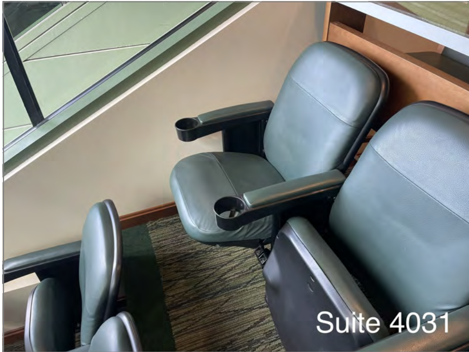
Interior and Finishes: Photo 4-4-16 Chair seat does not automatically close
