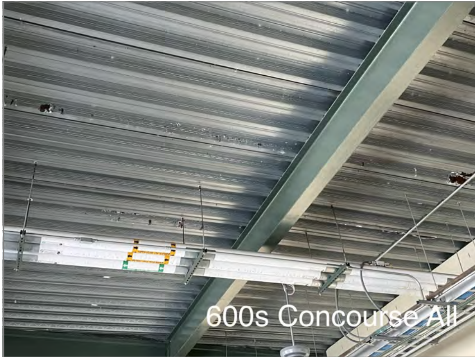
Concourses: Photo 2-600-7 Corroding floor pan
