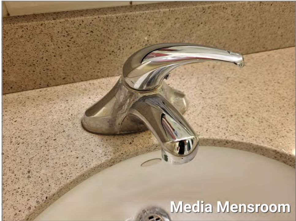
Plumbing: Photo 9- -1 Faucet leaking
