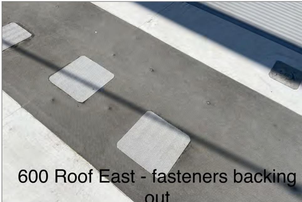
Roof: Photo 6- -19 Loose/backing out fastener
