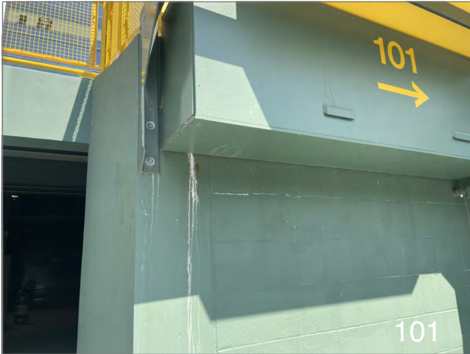
Bowl and Seating: Photo 1-2-62 Block cracking
