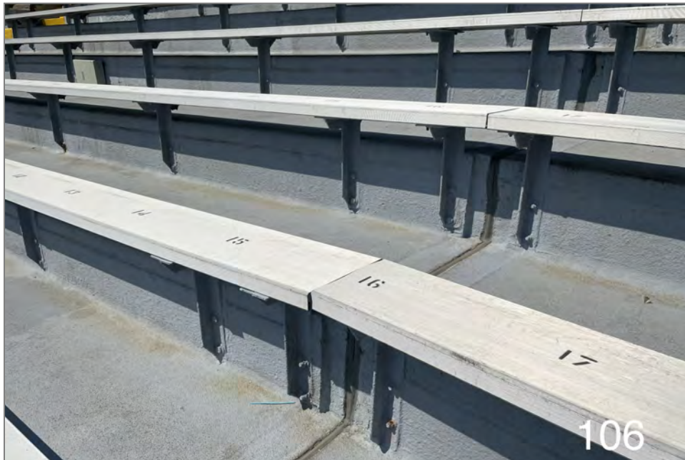
Bowl and Seating: Photo 1-2-78 Exposed expansion joint
