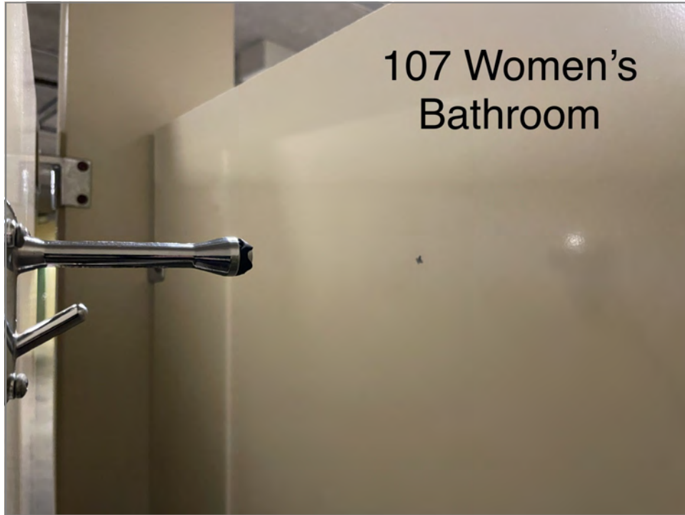
Interior and Finishes: Photo 4-5-10 Bathroom stall damaged
