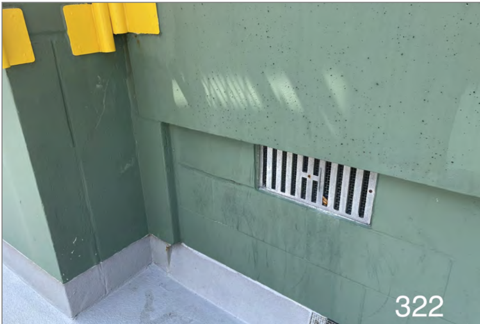
Bowl and Seating: Photo 1-2-87 Block cracking
