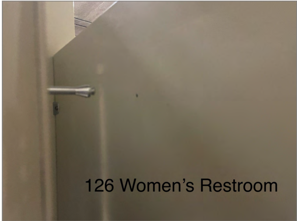
Interior and Finishes: Photo 4-5-19 Bathroom stall damaged
