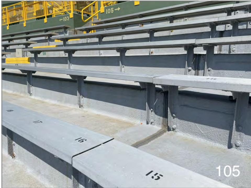
Bowl and Seating: Photo 1-2-75 Exposed expansion joint
