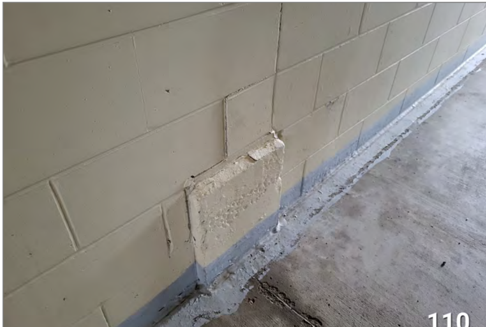
Concourses: Photo 2-100-16 Block cracking
