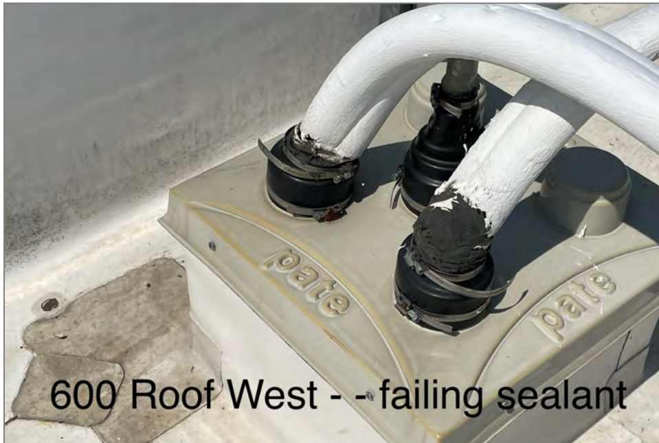
Roof: Photo 6- -32 Sealant deterioration
