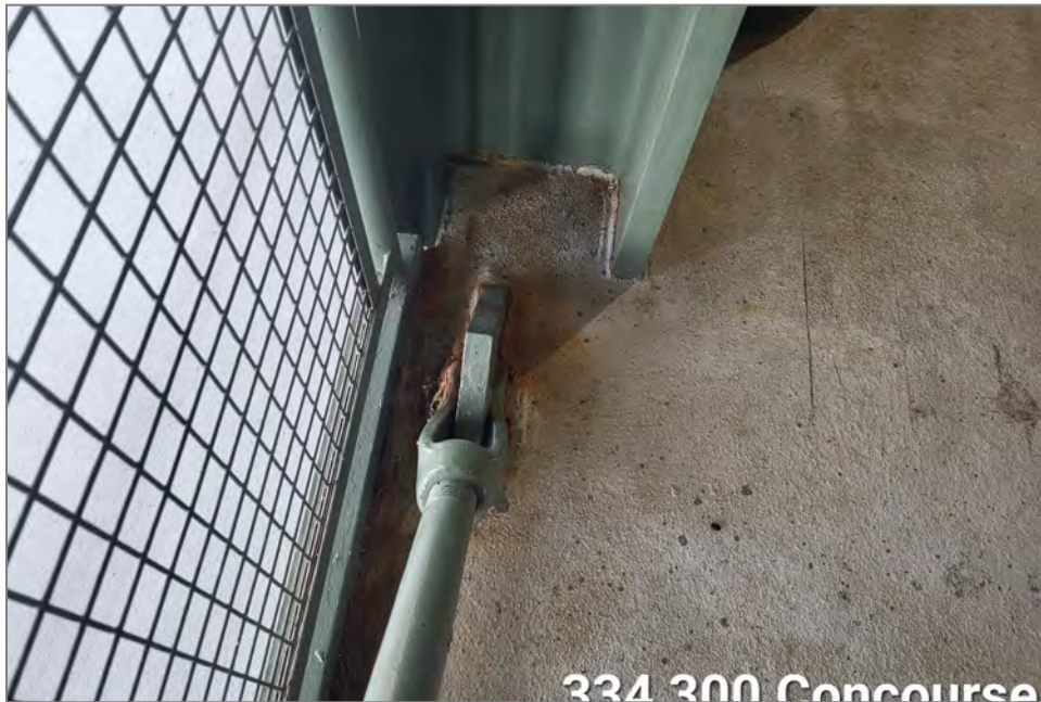
Concourses: Photo 2-300-6 Structural steel corrosion
