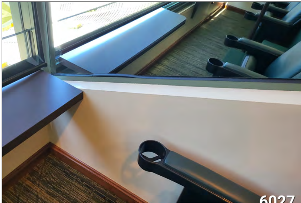
Interior and Finishes: Photo 4-4-13 Window frame seal failing
