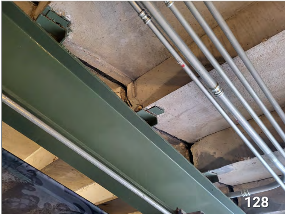
Concourses: Photo 2-100-18 Precast concrete spalling
