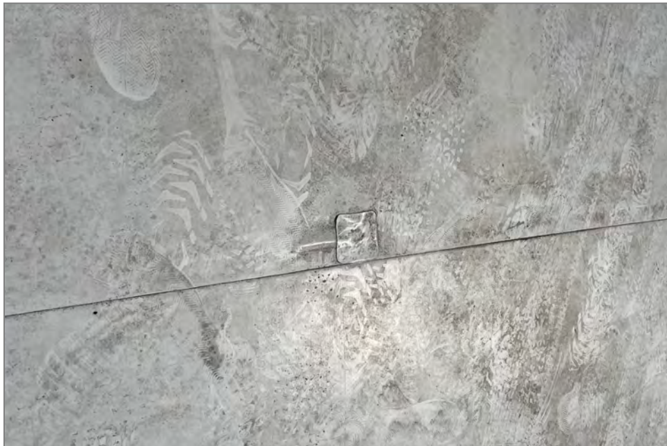
Roof: Photo 6- -17 Failing patch
