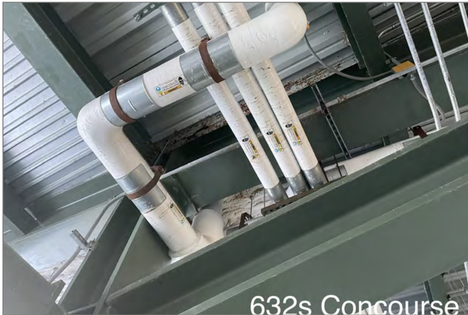
Concourses: Photo 2-600-5 Corroding floor pan
