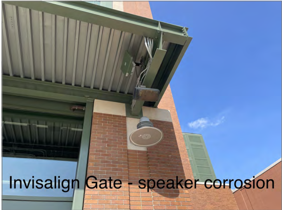
Exterior Walls: Photo 5- -12 Exterior speaker corrosion
