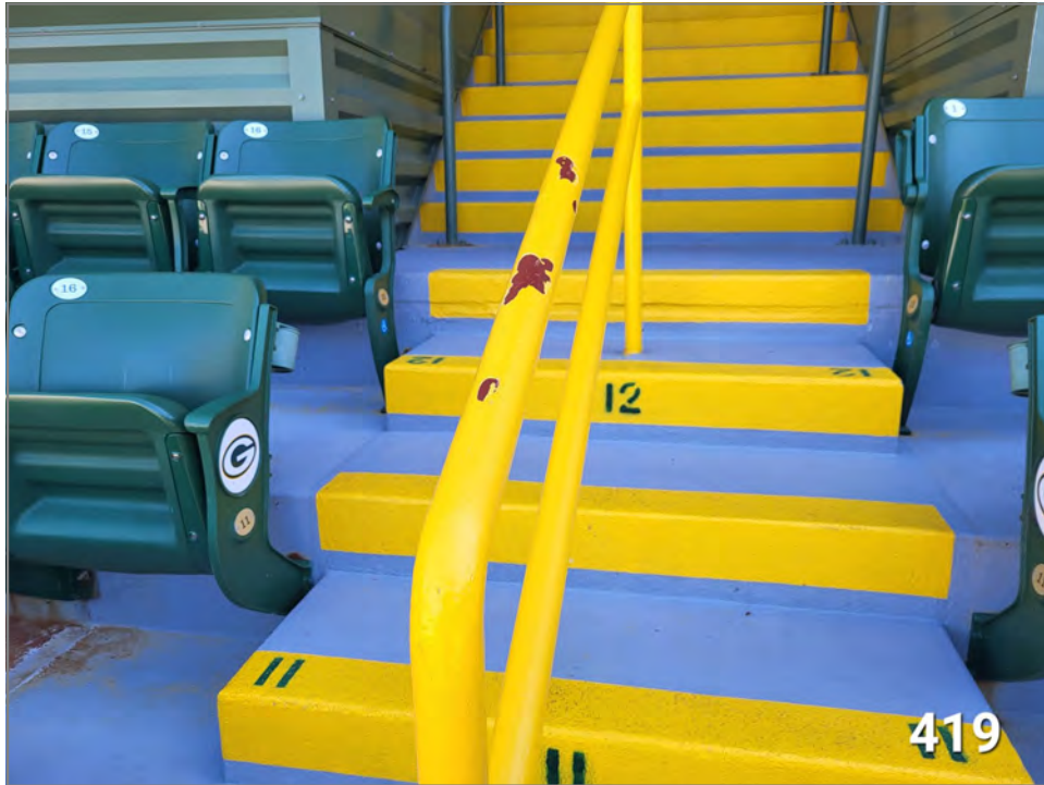
Bowl and Seating: Photo 1-2-25 Paint peeling/cracking or bubbling
