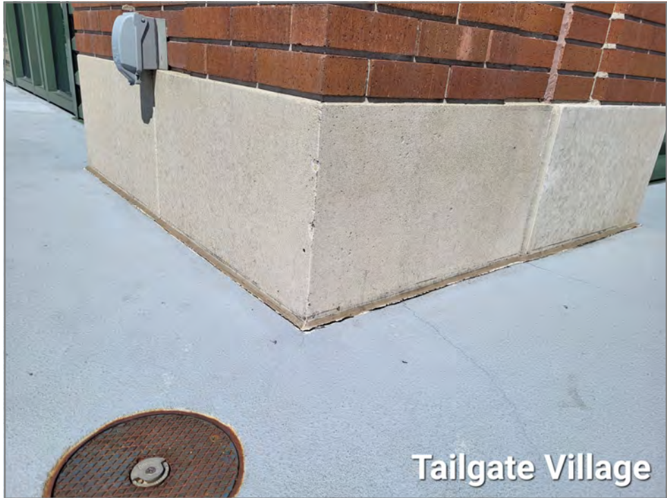
Site: Photo 10-1-4 Sealant failing
