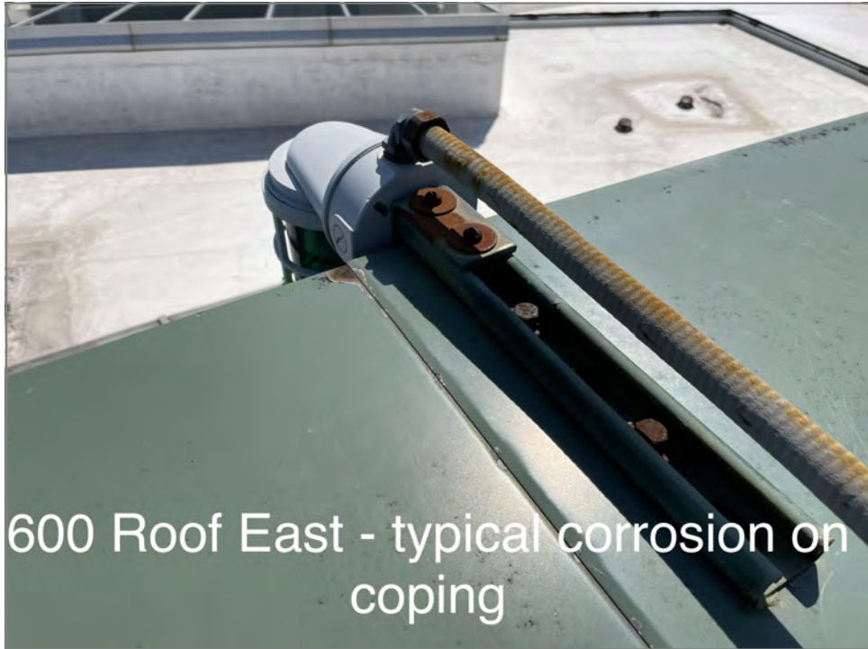
Roof: Photo 6- -18 Coping corrosion
