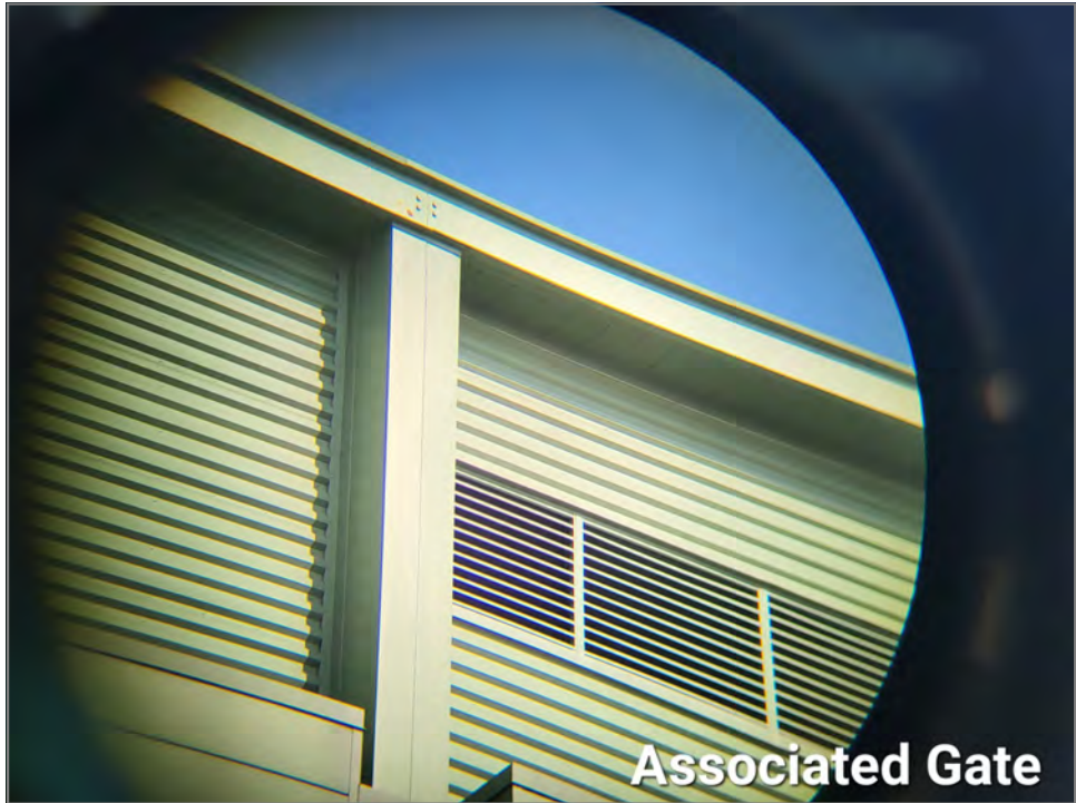
Exterior Walls: Photo 5- -2 Corrosion
