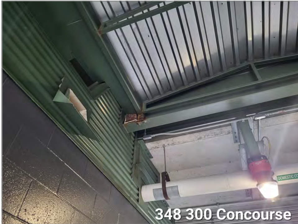
Concourses: Photo 2-300-4 Structural steel corrosion
