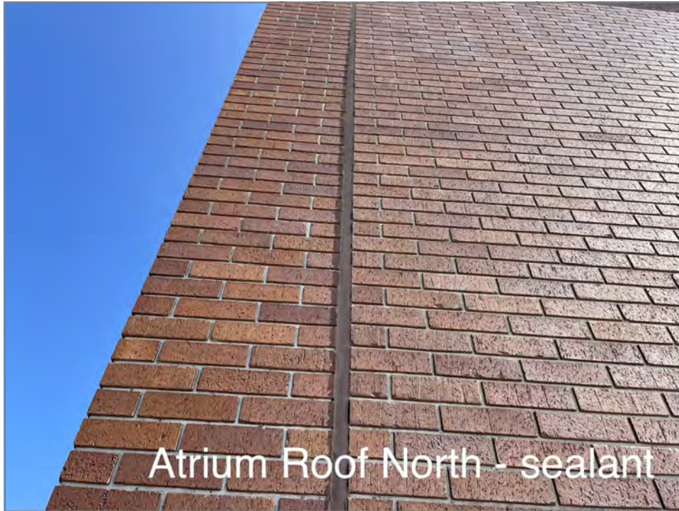
Roof: Photo 6- -12 Sealant deterioration
