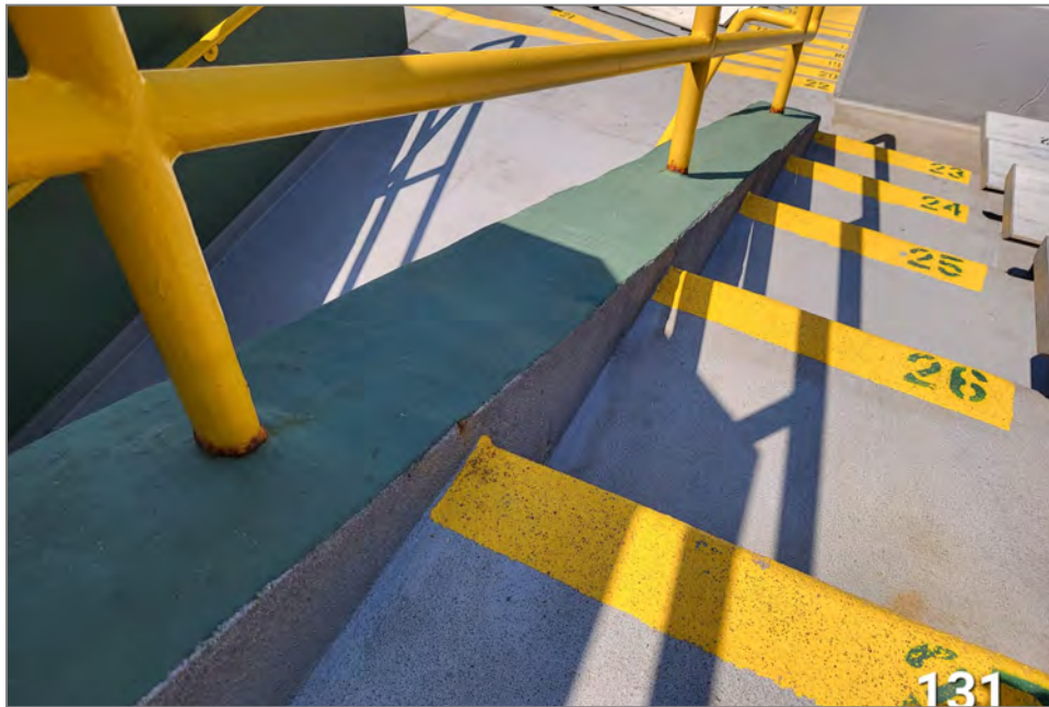
Bowl and Seating: Photo 1-2-10 Handrail and base corrosion
