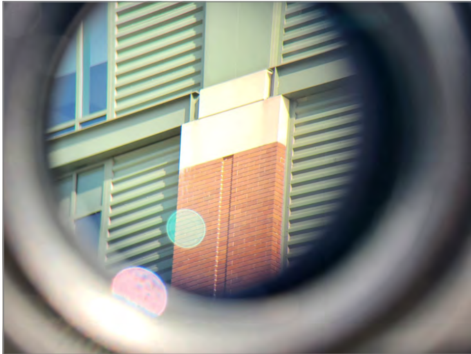
Exterior Walls: Photo 5--7 Efflorescence/staining
