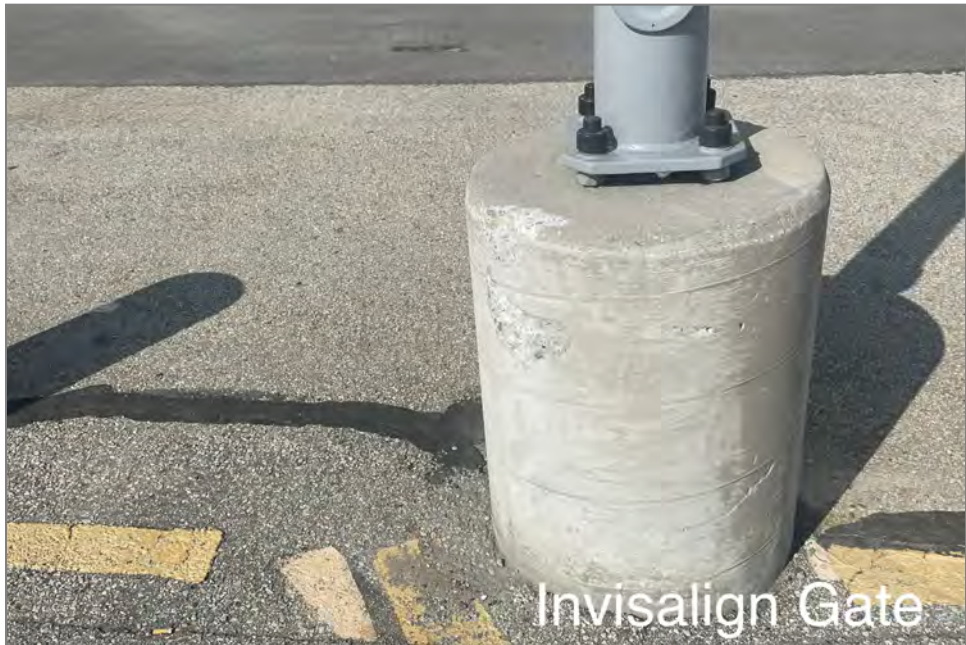
Site: Photo 10- -8 Light pole base damaged
