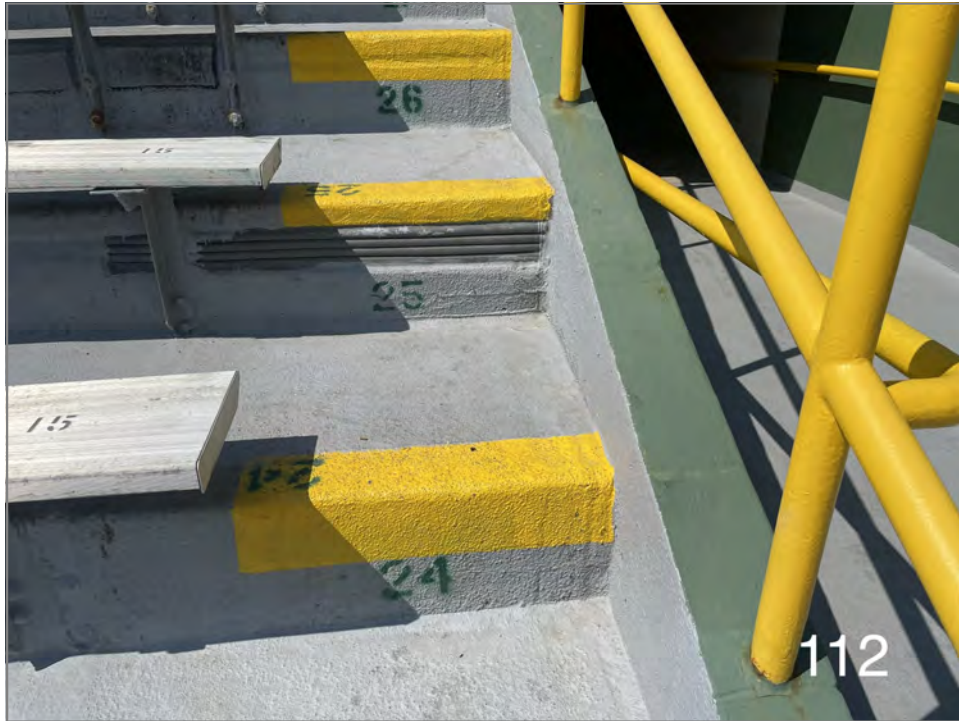
Bowl and Seating: Photo 1-2-64 Exposed expansion joint
