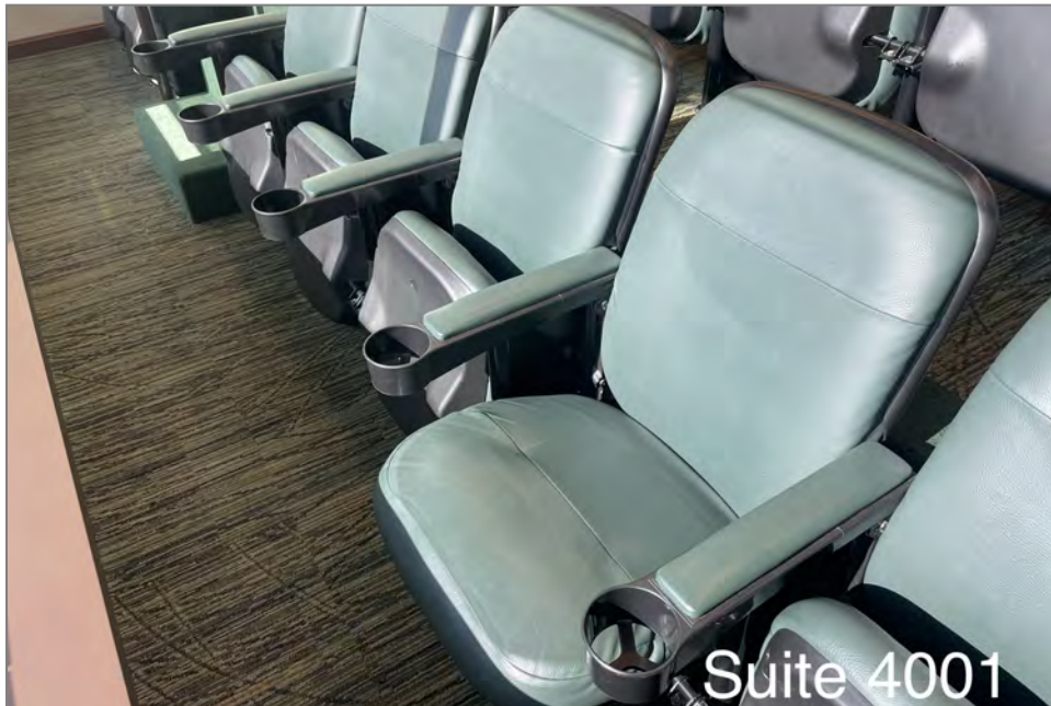
Interior and Finishes: Photo 4-4-27 Chair seat does not automatically close
