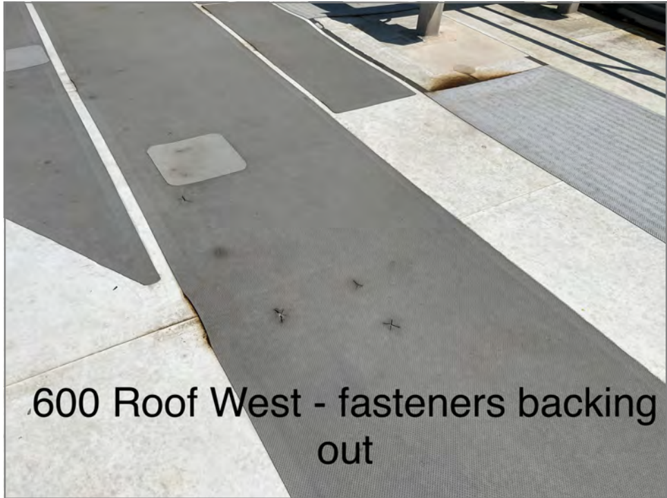
Roof: Photo 6- -33 Loose/backing out fastener
