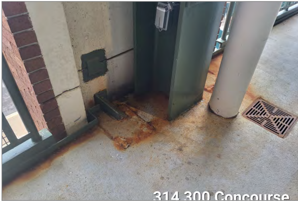
Concourses: Photo 2-300-8 Structural steel corrosion
