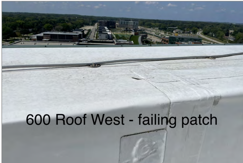
Roof: Photo 6- -31 Failing patch
