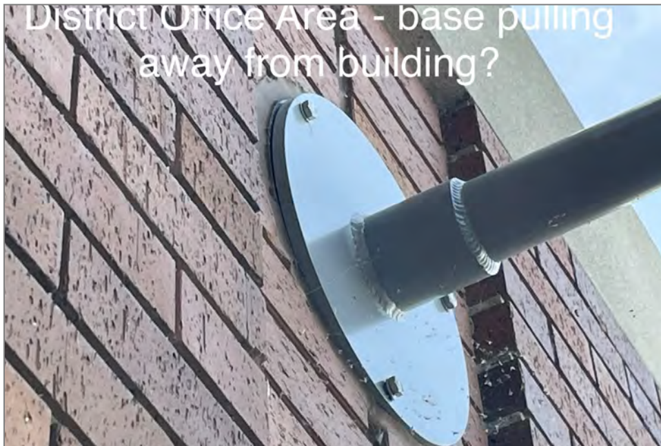
Exterior Walls: Photo 5- -22 Fixture loose
