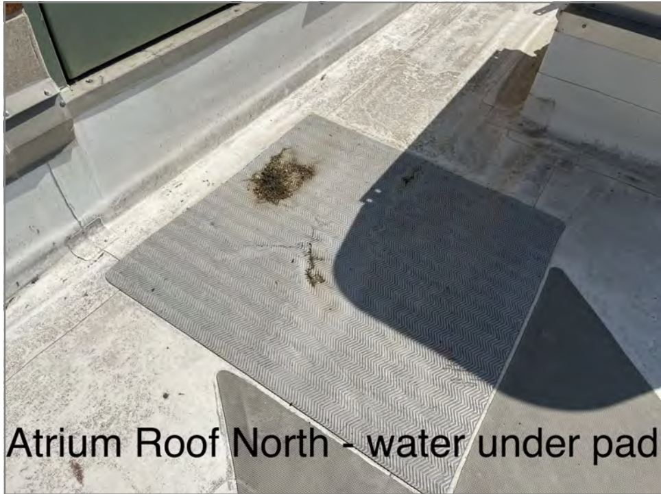
Roof: Photo 6- -13 Water under pad
