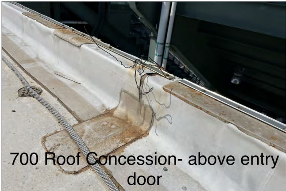
Roof: Photo 6- -36 Membrane cut/open
