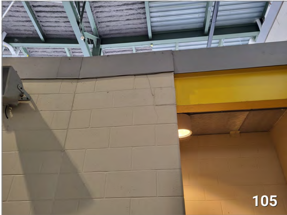
Concourses: Photo 2-100-9 Block cracking
