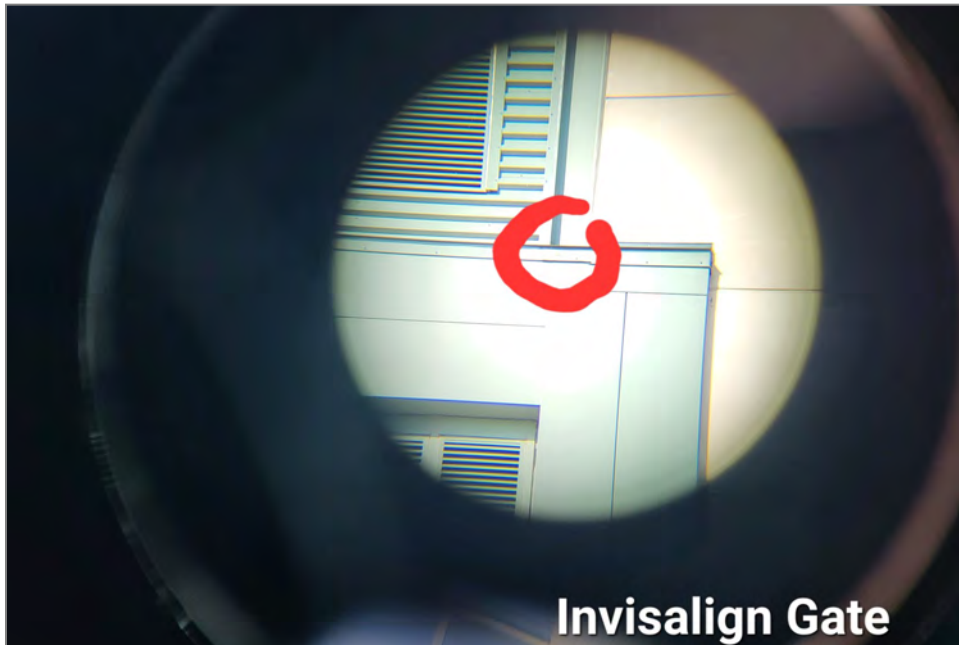
Exterior Walls: Photo 5--01 Missing/failing sealant
