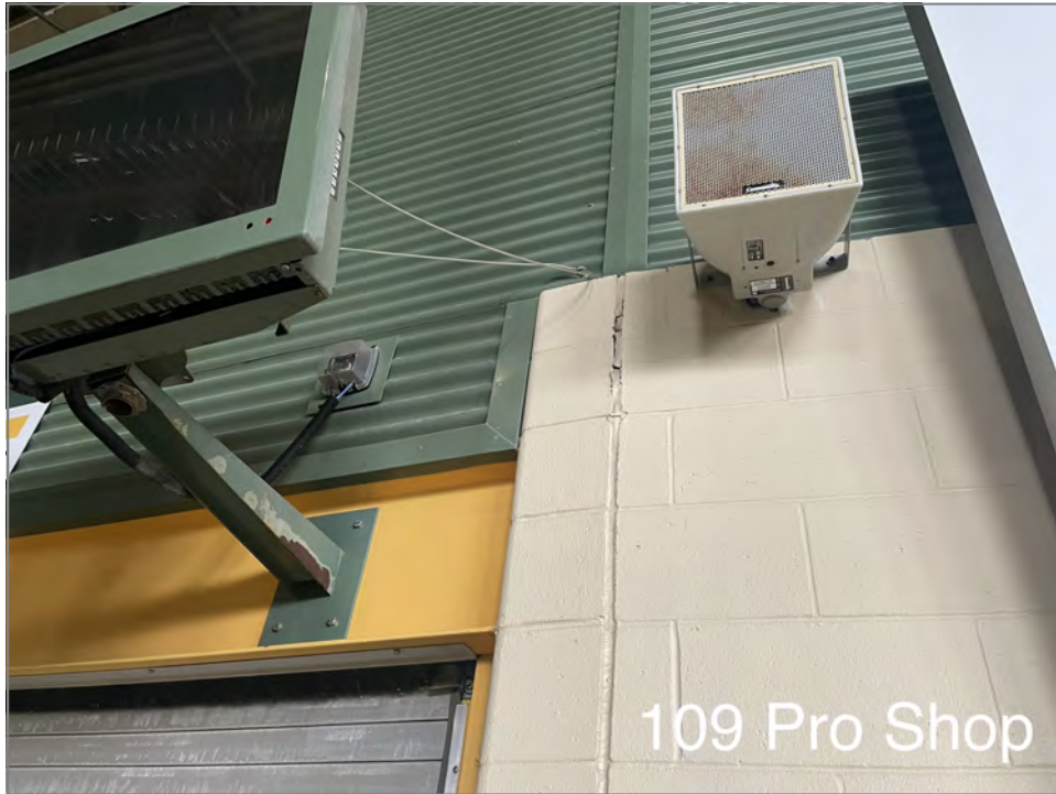
Concourses: Photo 2-100-30 Sealant failing
