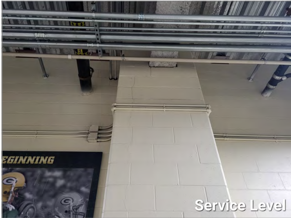
Concourses: Photo 2-0-2 Block cracking
