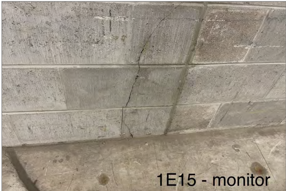
Miscellaneous: Photo 11- -1 Cracking CMU—Monitor
