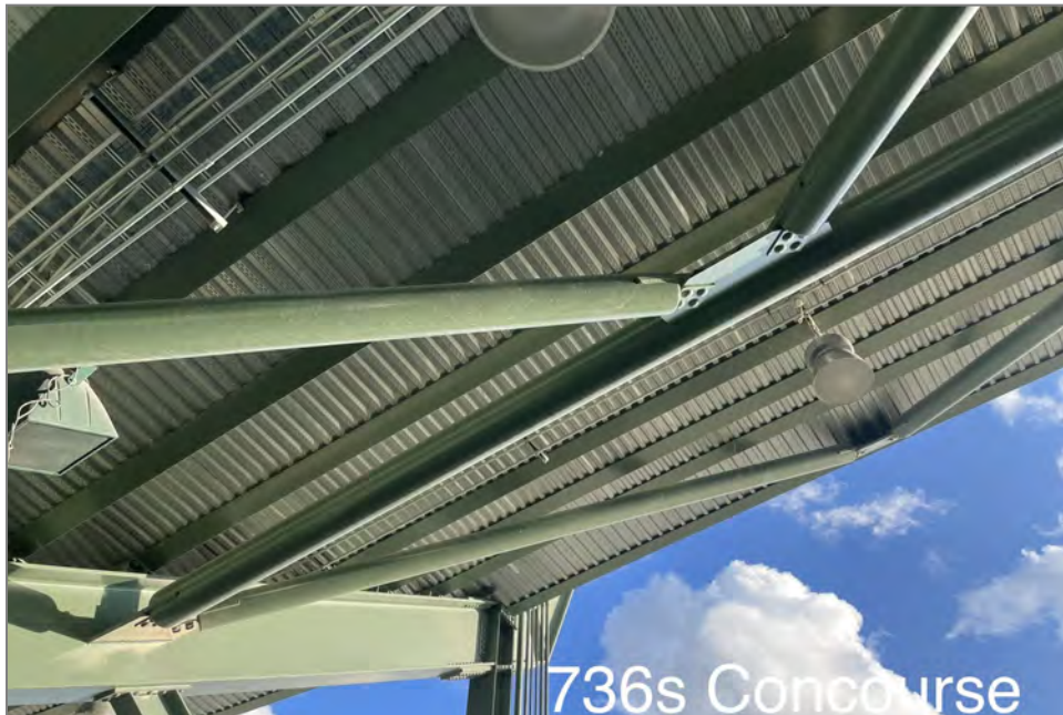
Concourses: Photo 2-700-3 Corroding floor pan
