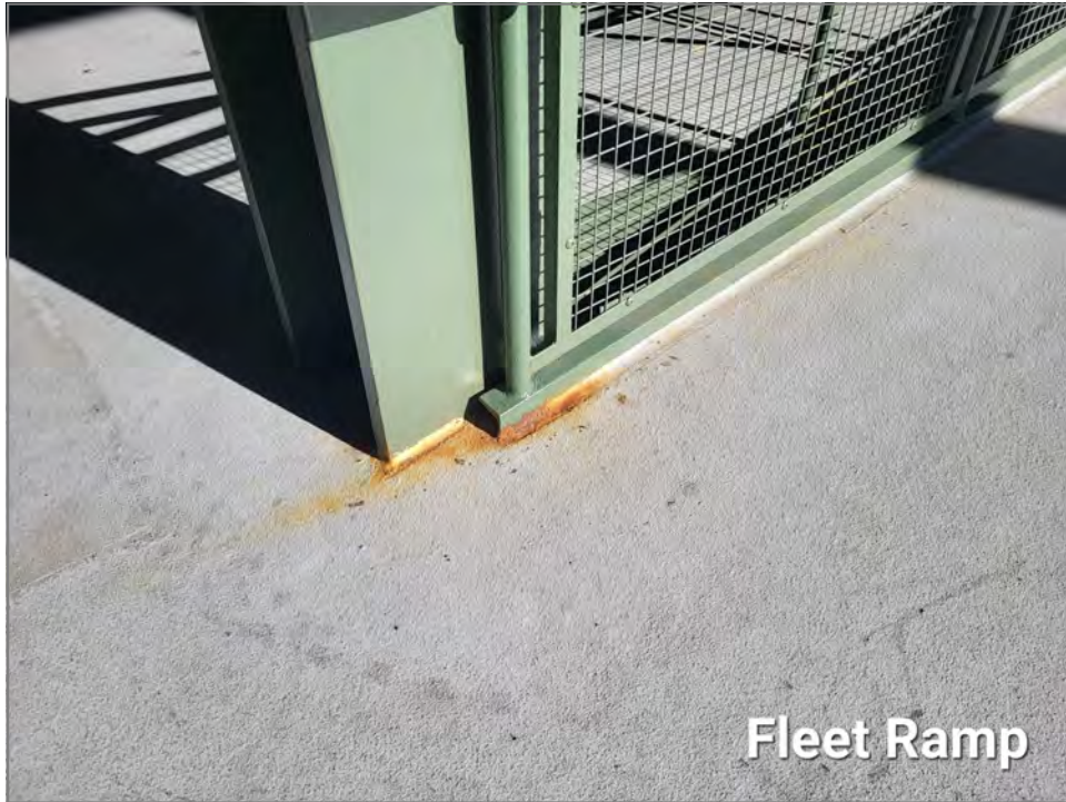
Concourses: Photo 2-900-3 Handrail corrosion
