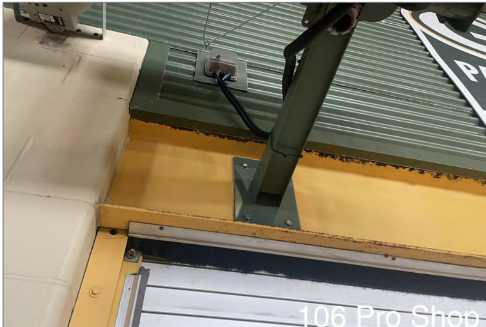
Concourses: Photo 2-100-32 Paint peeling
