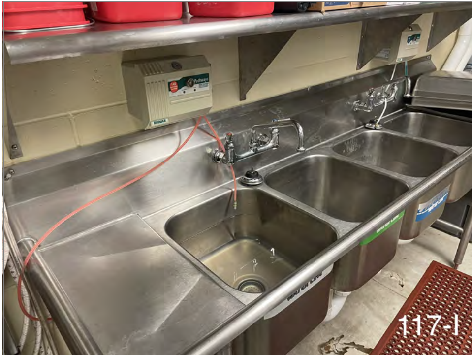
Concessions: Photo 3- -5 Sink improperly draining
