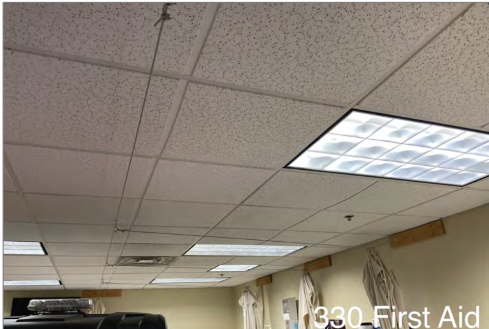
Interior and Finishes: Photo 4- - 10 Sagging drop ceiling grid
