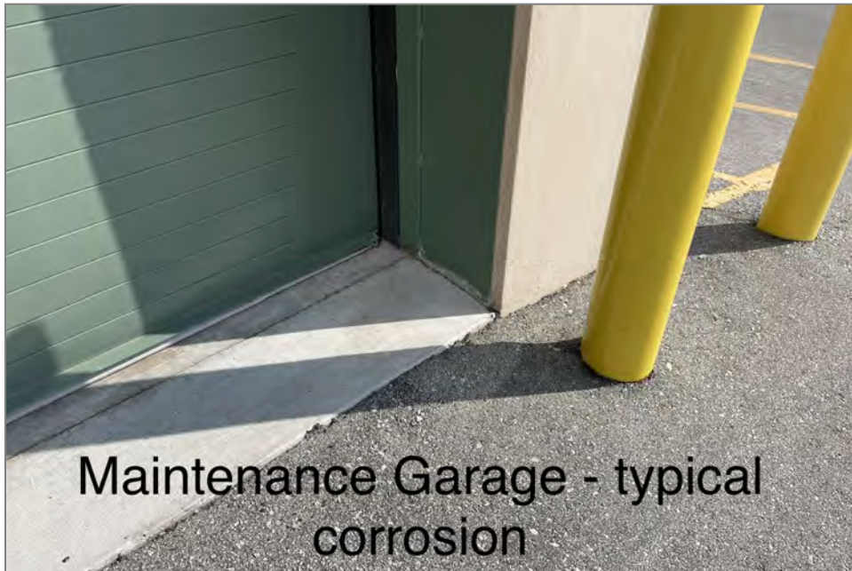
Exterior Walls: Photo 5- -10 Corrosion
