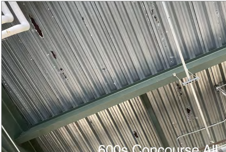
Concourses: Photo 2-600-9 Corroding floor pan
