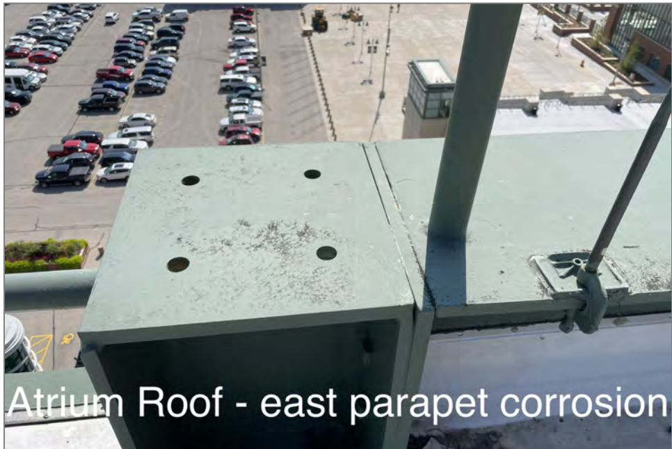
Roof: Photo 6- -14 Corrosion on parapet/rail
