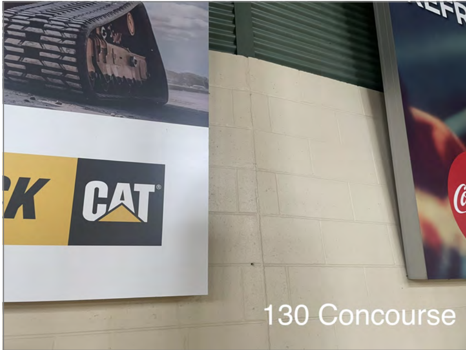
Concourses: Photo 2-100-34 Sealant failing
