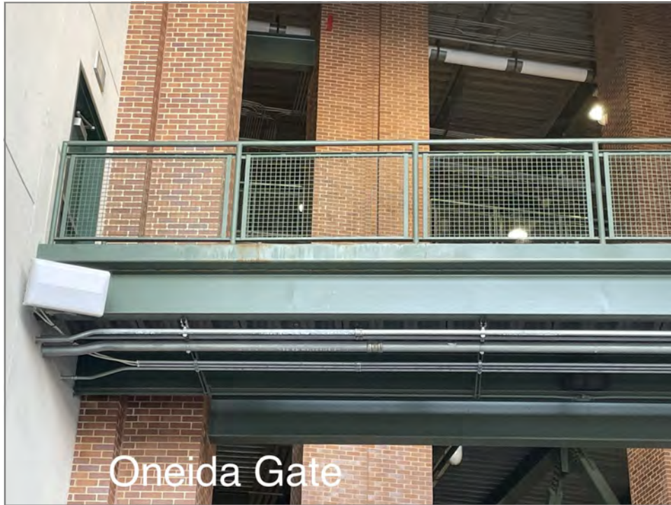
Exterior Walls: Photo 5- -32 Corrosion
