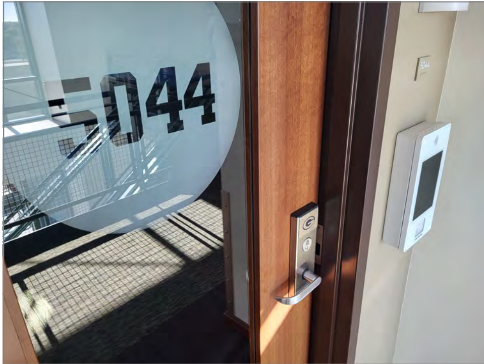
Interior and Finishes: Photo 4-4-9 Door won't close automatically
