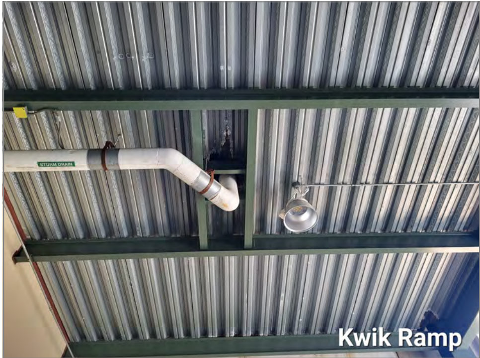
Concourses: Photo 2-900-1 Floor pan corroding
