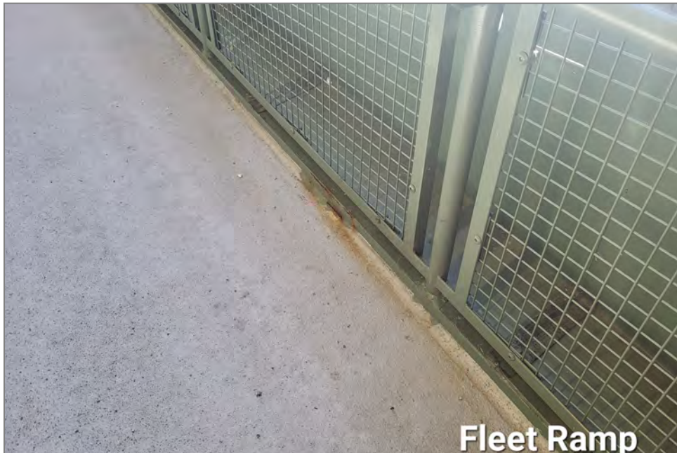
Concourses: Photo 2-900-2 Handrail corrosion
