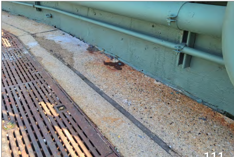
Bowl and Seating: Photo 1-1-6 Sealant failing
