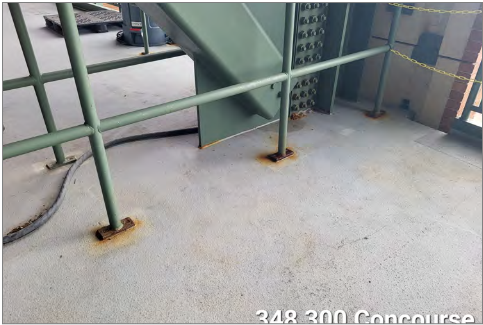
Concourses: Photo 2-300-3 Handrail and base corrosion
