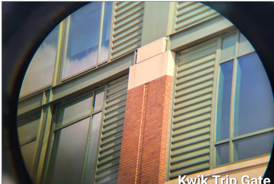
Exterior Walls: Photo 5--8 Efflorescence/staining
