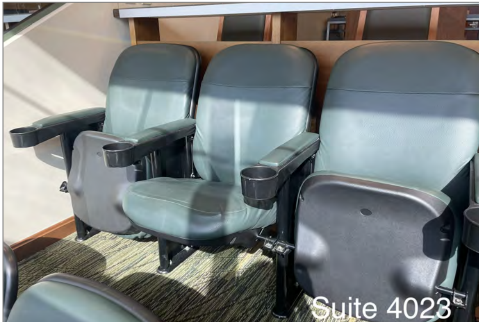
Interior and Finishes: Photo 4-4-20 Chair seat does not automatically close
