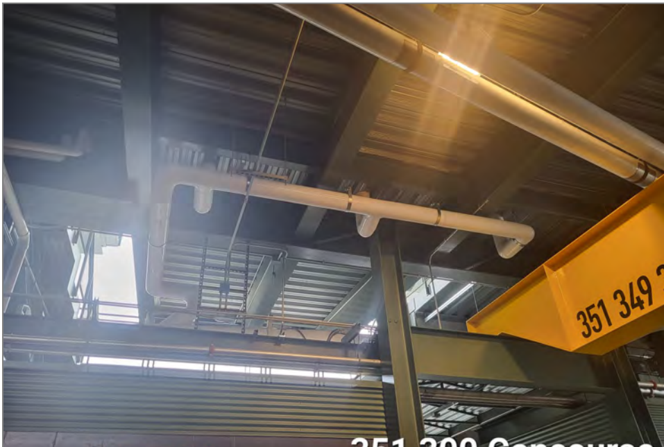
Concourses: Photo 2-300-1 Missing saddle plates
