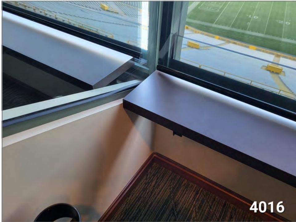
Interior and Finishes: Photo 4-4-6 Window frame seal failing
