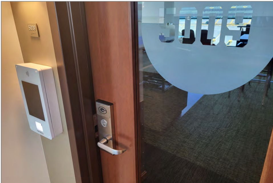
Interior and Finishes: Photo 4-4-7 Door won't close automatically
