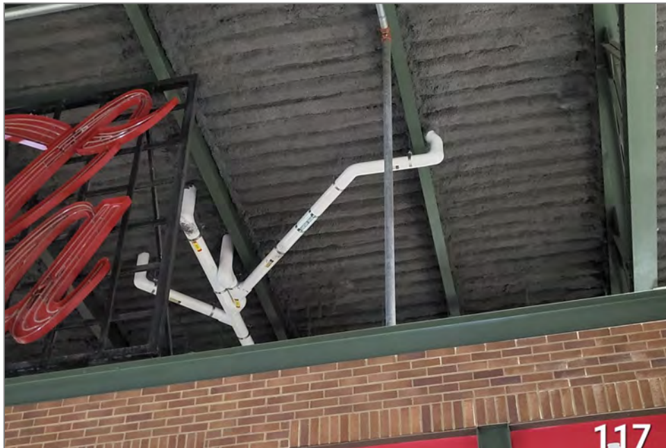
Concourses: Photo 2-100-5 Missing saddle plates
