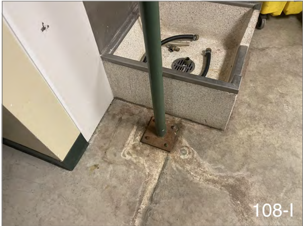
Concessions: Photo 3- -13 Handrail and base corrosion
