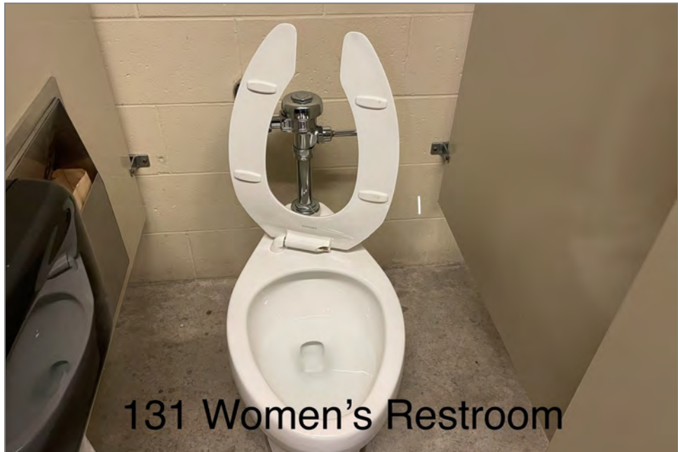
Interior and Finishes: Photo 4-5-23 Toilet seat broken
