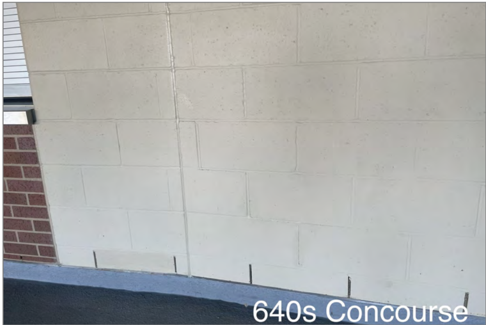
Concourses: Photo 2-600-10 Block cracking
