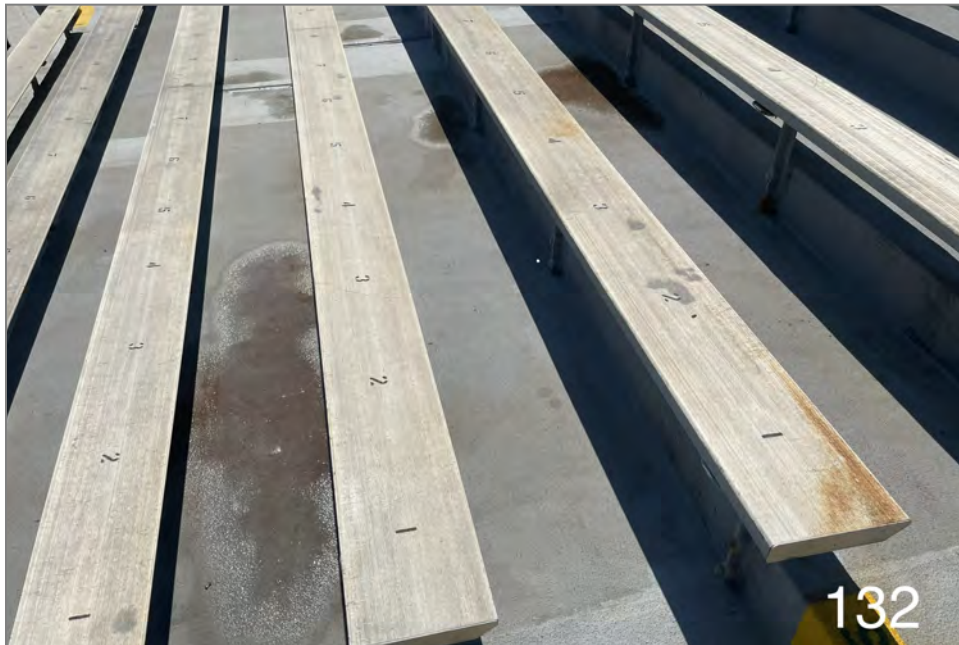
Bowl and Seating: Photo 1-2-53 Bleachers corroding
