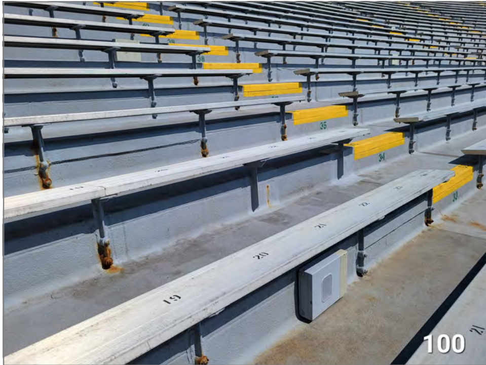
Bowl and Seating: Photo 1-2-6 Bleacher support corroding
