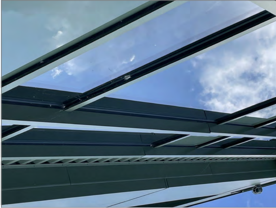
Exterior Walls: Photo 5- -34 Mullions shifting/misaligned
