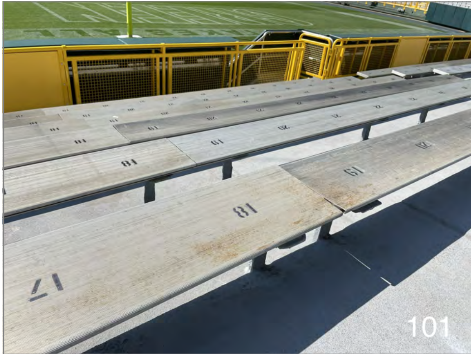
Bowl and Seating: Photo 1-2-49 Bleachers corroding
