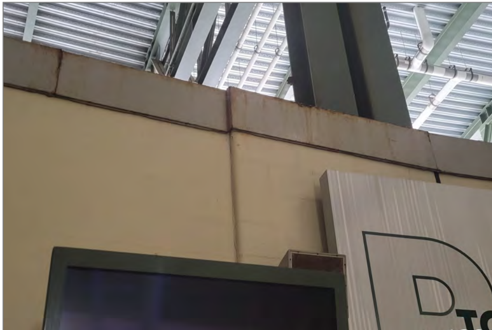
Concourses: Photo 2-100-24 Flashing corroding
