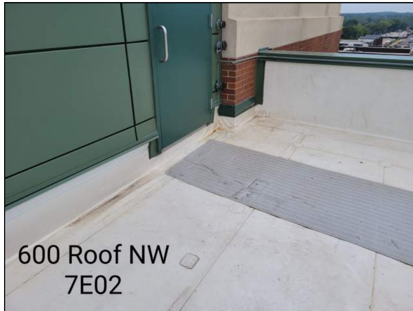
Roof: Photo 6- -12 Decking/Insulation Deterioration
