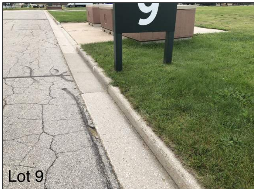
Site: Photo 10- -19 Pavement Cracking
