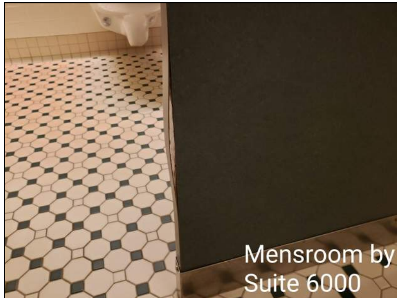
Interior and Finishes: Photo 4-5-19 Stall Damaged
