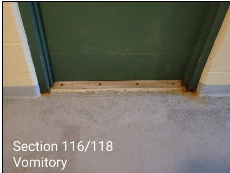
Concourses: Photo 2-100-55 Door Frame Corrosion
