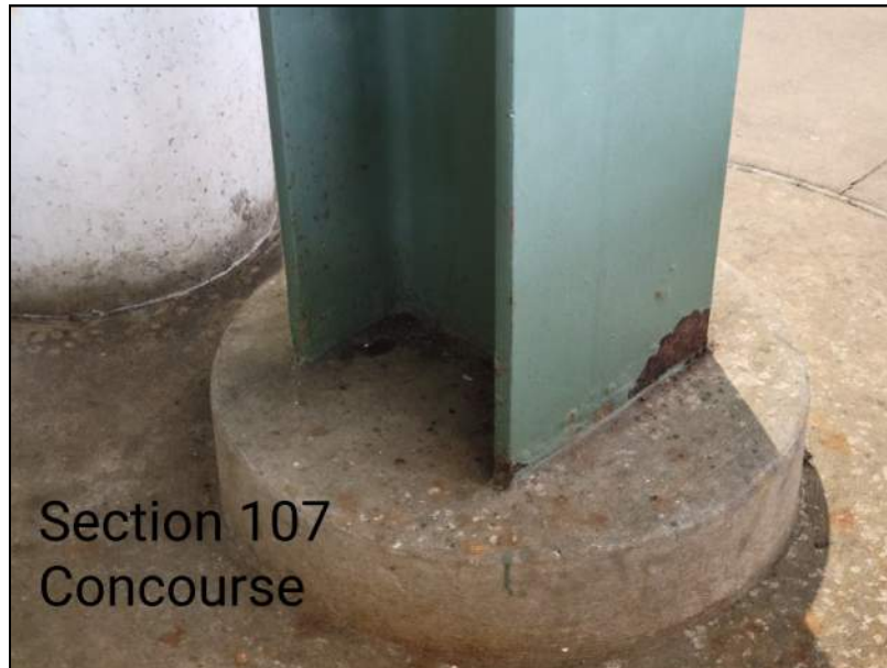
Concourses: Photo 2-100-25 Structural Steel Corrosion
