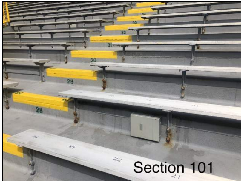
Bowl and Seating: Photo 1- -151 Corrosion
