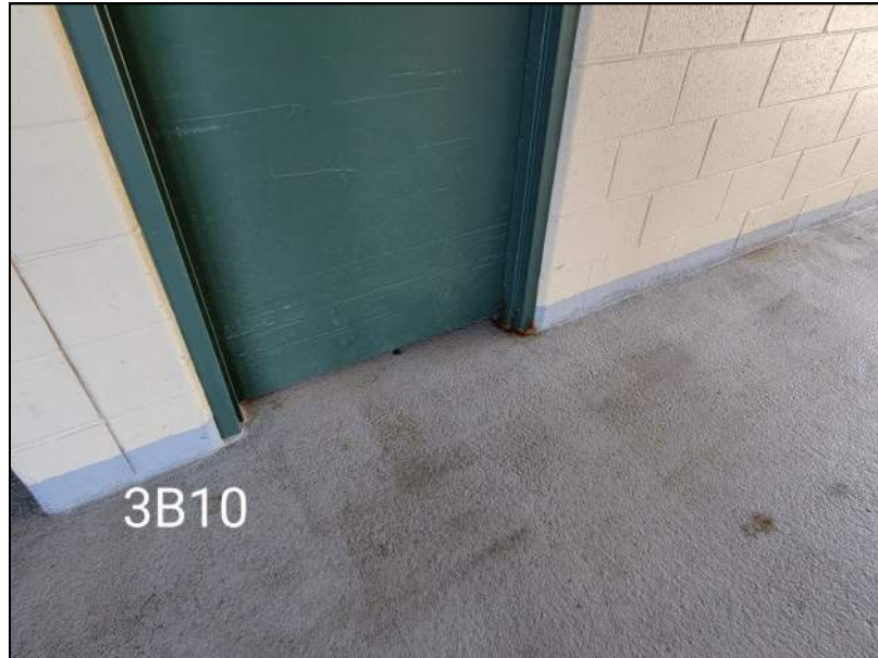
Concourses: Photo 2-300-12 Door Frame Corrosion
