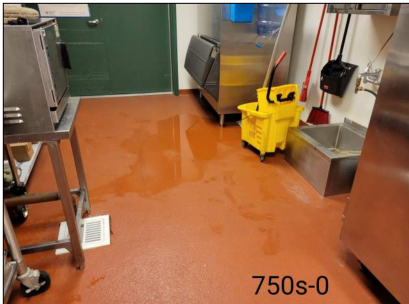
Concessions: Photo 3- -1 Ice Machine Leaking
