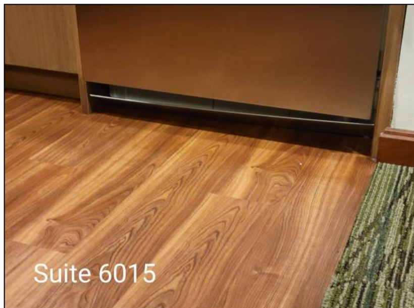
Interior and Finishes: Photo 4-4-8 Appliance Damage
