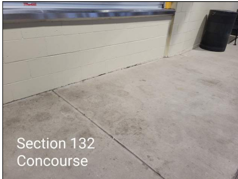
Concourses: Photo 2-100-62 Mortar Deteriorating
