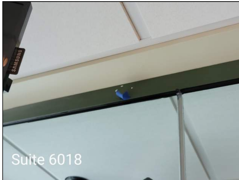
Interior and Finishes: Photo 4-4-11 Window Frame Damage
