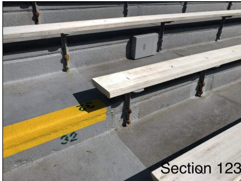
Bowl and Seating: Photo 1- -45 Corrosion
