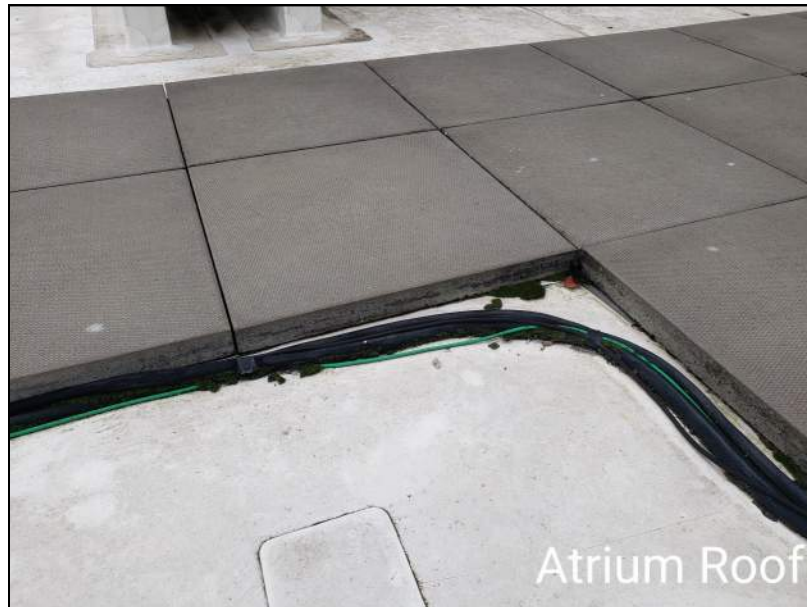
Roof: Photo 6- -1 Biological Growth
