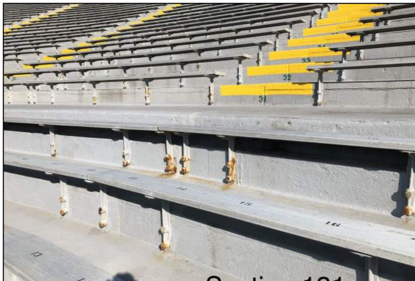
Bowl and Seating: Photo 1- -91 Corrosion
