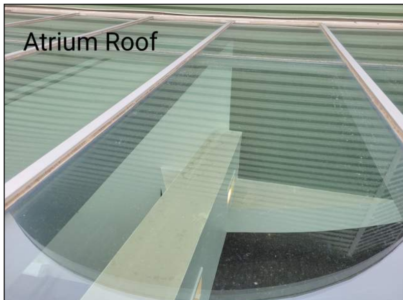
Roof: Photo 6- -7 Prior Leaks
