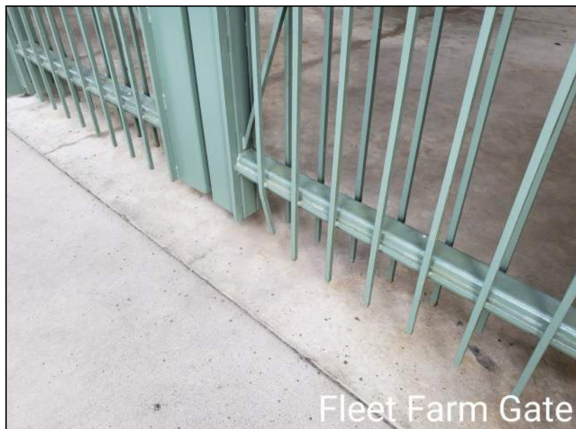
Exterior Walls: Photo 5- -8 Gate Damaged
