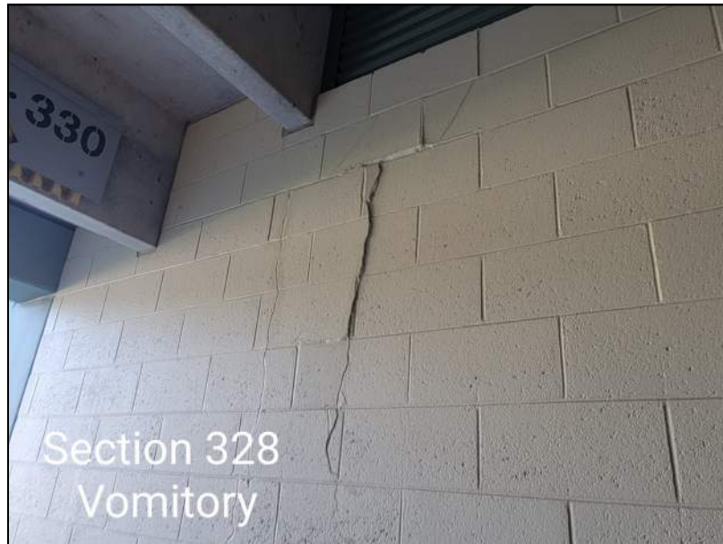
Concourses: Photo 2-300-35 Concrete Block Damage
