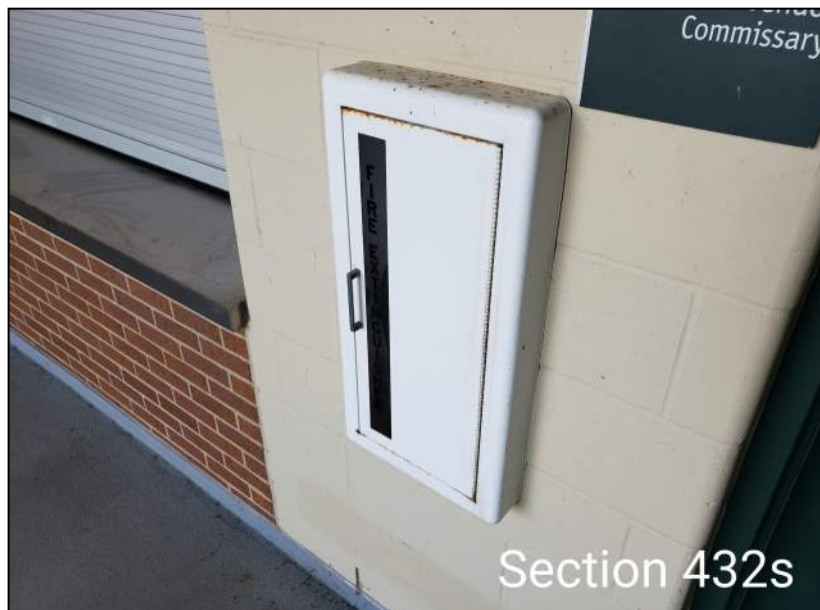
Concourses: Photo 2-400-3 Fire Extinguisher Cabinet Corrosion
