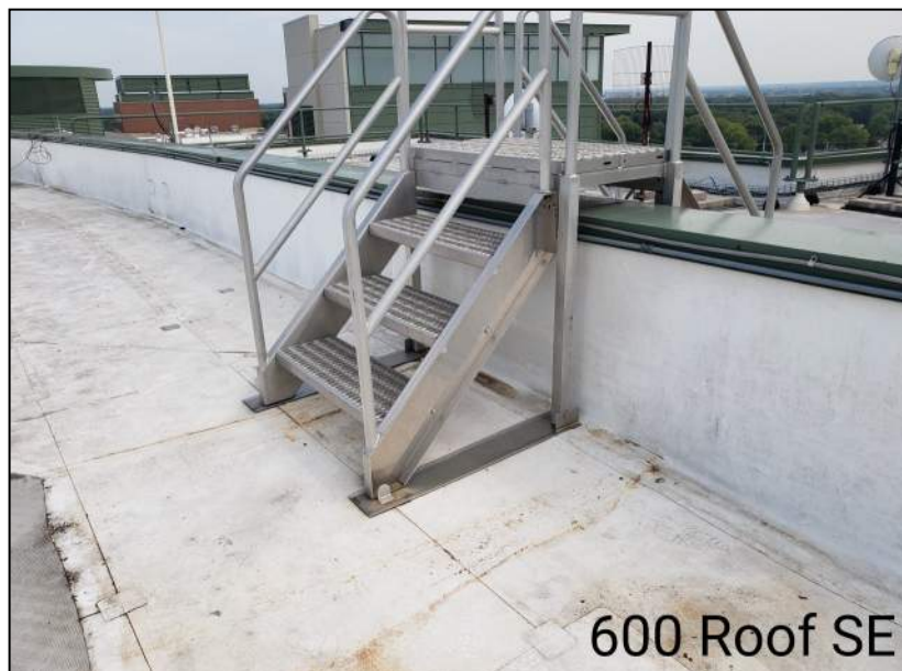
Roof: Photo 6- -24 Missing Slip Sheet
