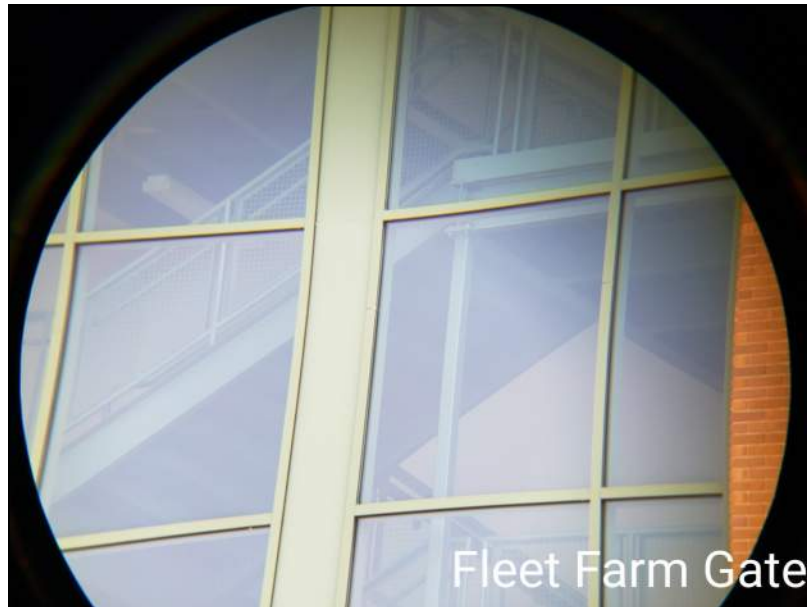
Exterior Walls: Photo 5- -6 Window Mullion Failing
