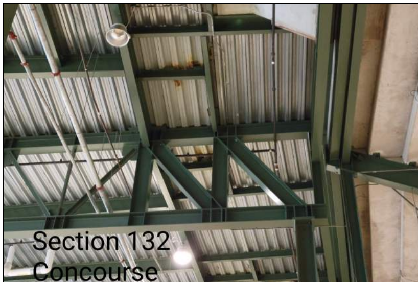
Concourses: Photo 2-100-65 Floor Pan Corrosion
