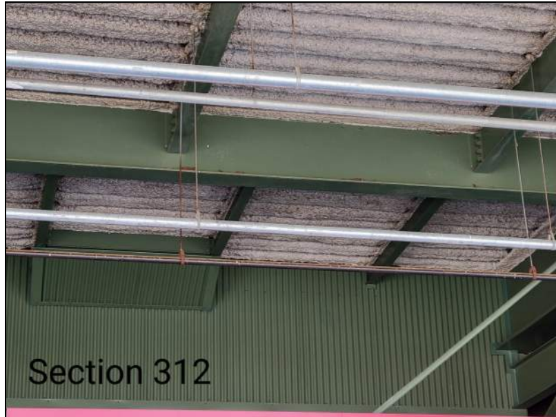
Concourses: Photo 2-300-1 Structural Steel Corrosion
