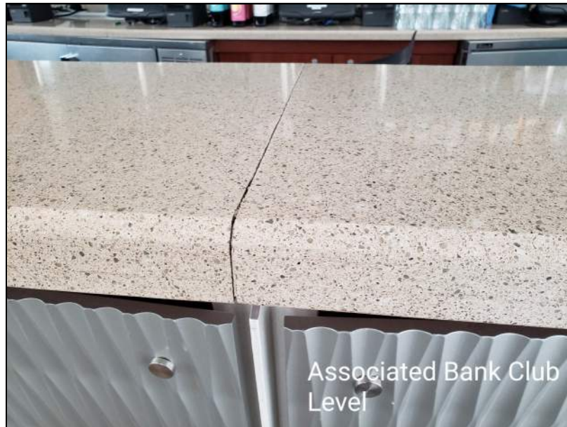
Concourses: Photo 2-400-11 Grout Deteriorating
