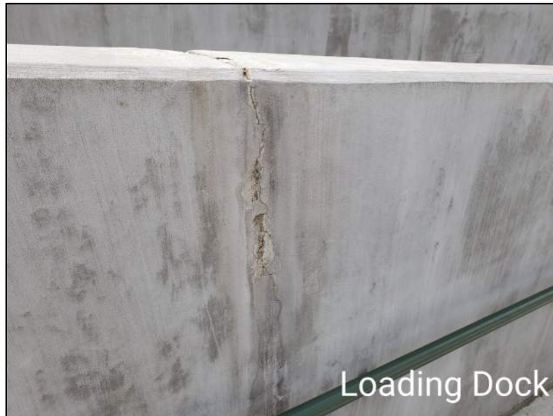
Site: Photo 10- -2 Concrete Spalling
